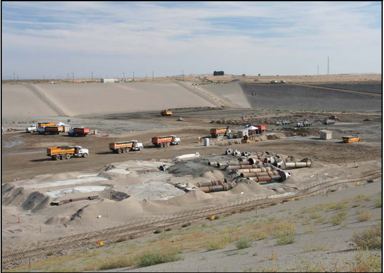
The Waste Operations team at the Environmental Restoration Disposal Facility has disposed of a record 2.1 million tons of waste so far this fiscal year. The previous record was 1.6 million tons, set last year. (Photo 1)
