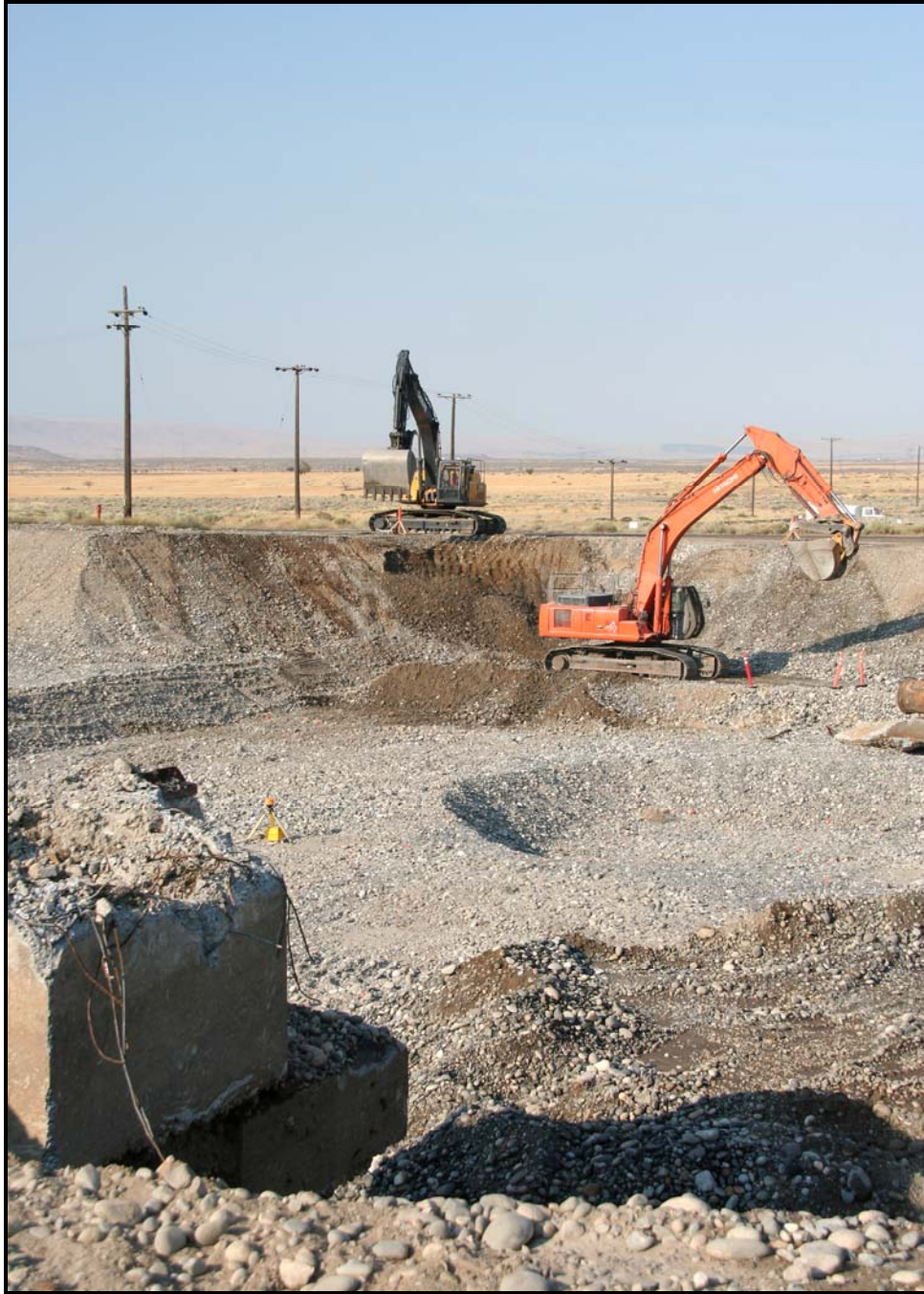
Washington Closure Hanford subcontractor Ojeda Business Ventures continues excavation at 100-F-57, a site that contains hexavalent chromium. (Photo 4)
