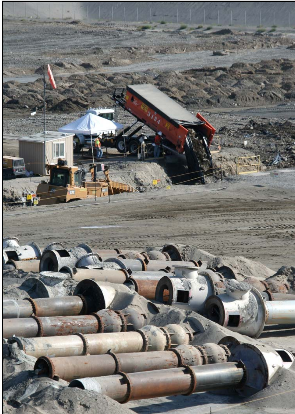
Waste material is dumped for disposal in super cell 10 at the Environmental Restoration Disposal Facility. In the foreground are pumps from the water intake structures at K Area. (Photo 2)
