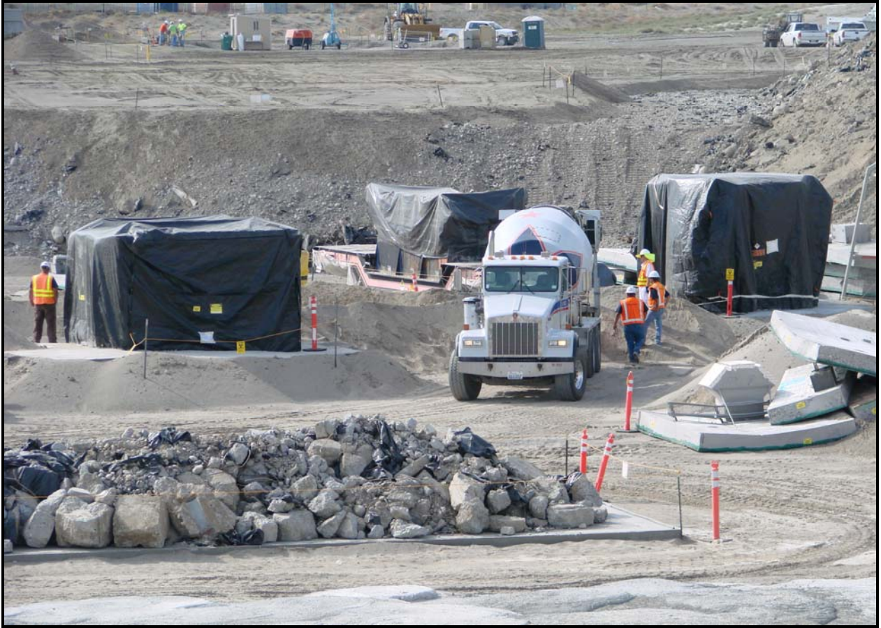
The Waste Operations team prepares to grout railcars for disposal at the Environmental Restoration Disposal Facility. (Photo 3)
