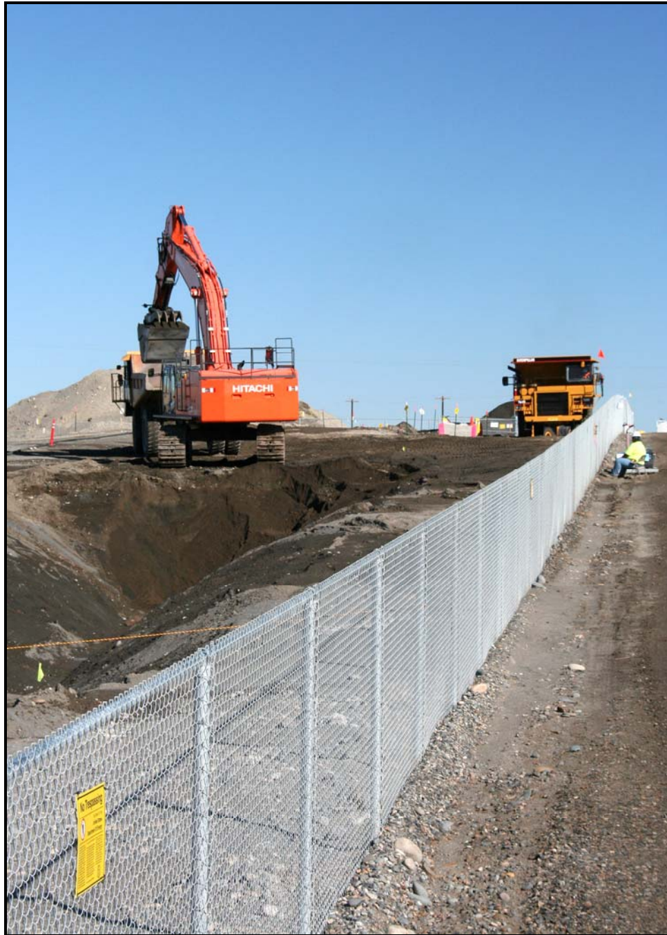
The surge trench on the east side of the 618-10 Burial Ground is expanded. Surge trenches are excavated in clean soil adjacent to the burial ground. They provide a below-ground area to hold material excavated during the trench excavation process. (Photo 6)
