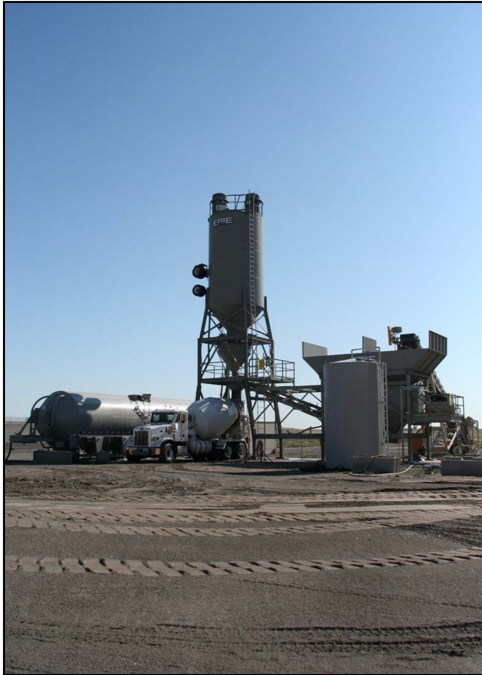
The new batch plant is producing grout material for disposal operations at the Environmental Restoration Disposal Facility. (Photo 3)
