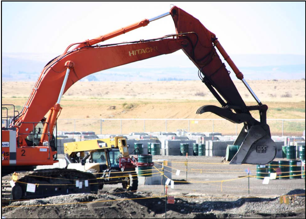
An excavator uncovers a concreted drum from the north trench of the 618-10 Burial Ground. (Photo 5)
