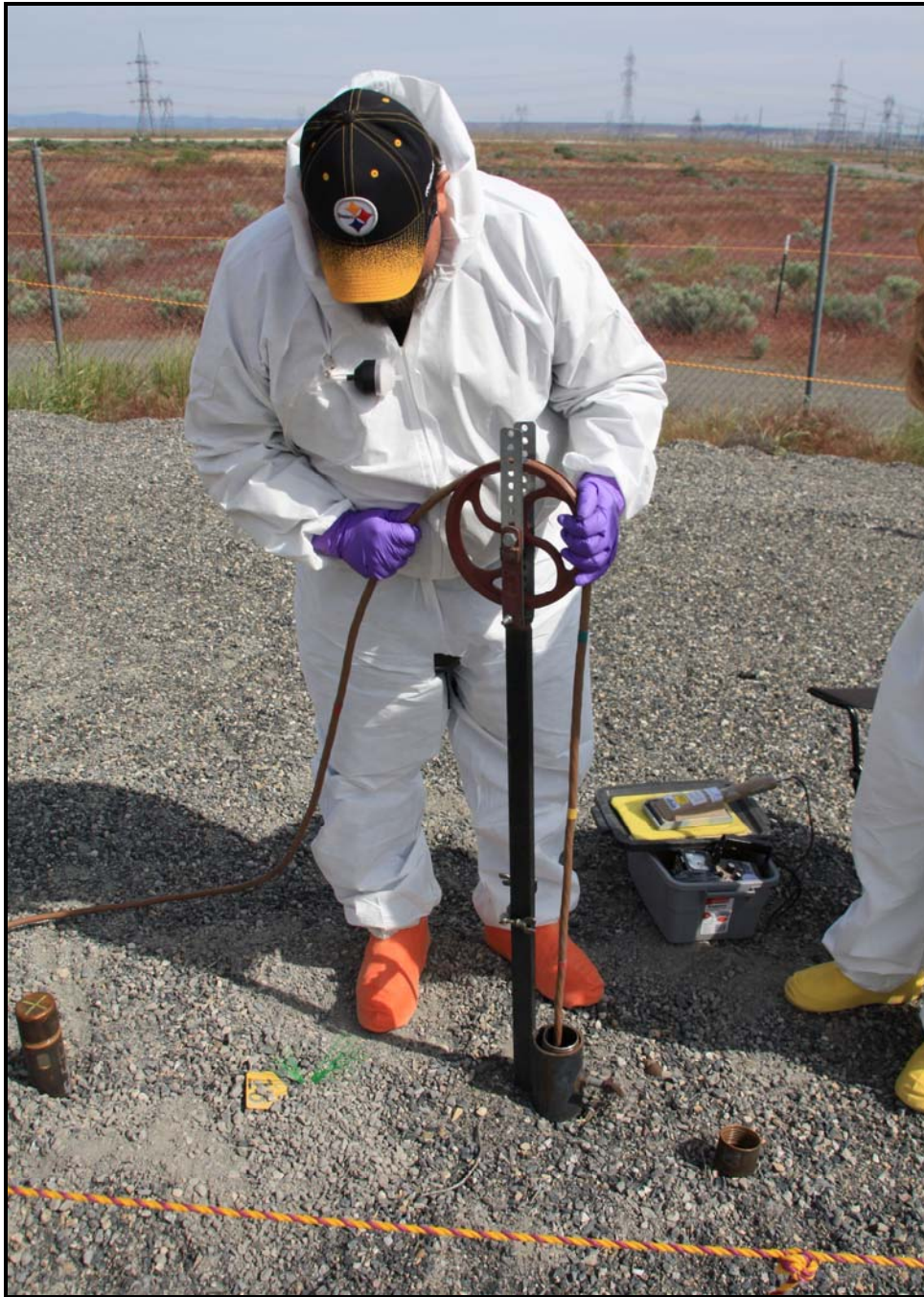
During nonintrusive characterization at the 618-11 Burial Ground, a multi-detector probe was used to identify the location of radioactive materials within the vertical pipe units. (Photo 7)
