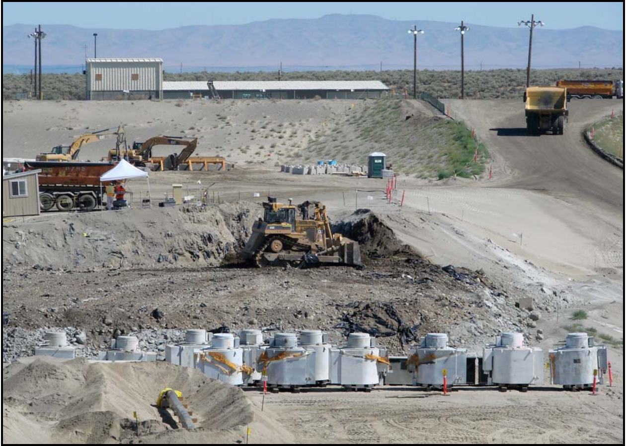
Motors for the pumps from the K reactors' water intake structures are being disposed at ERDF. (Photo 3)
