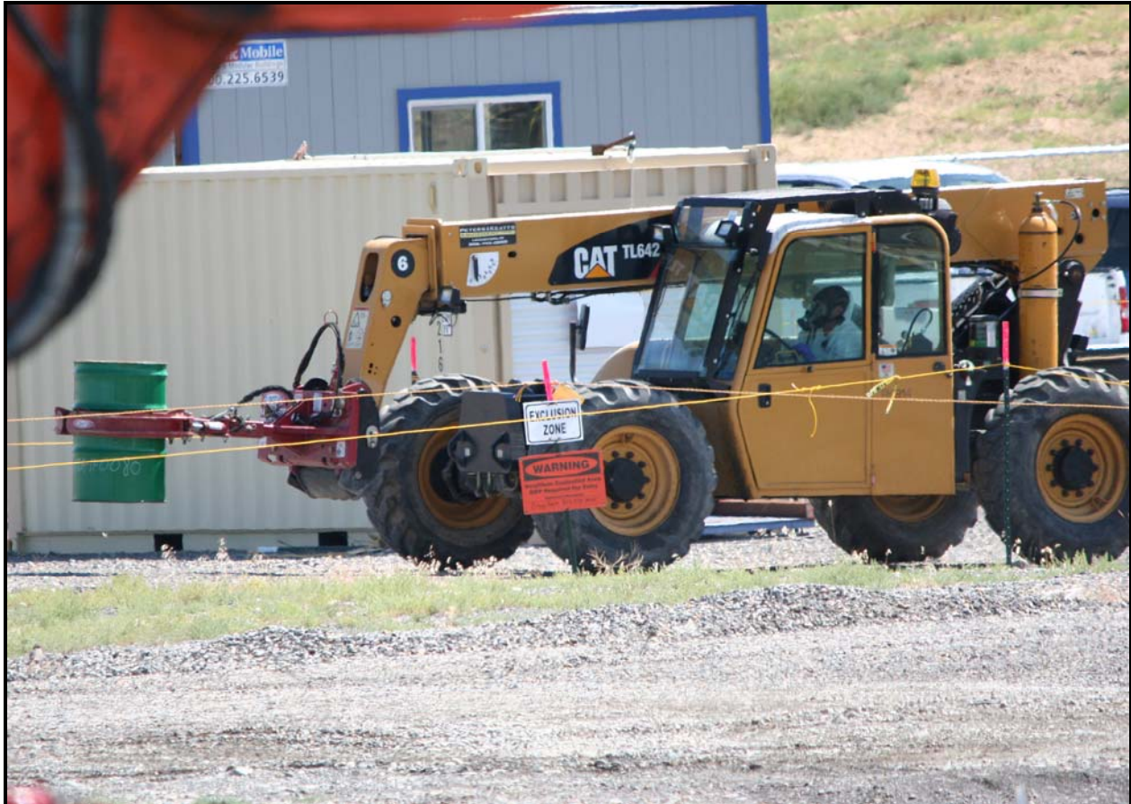
A telehandler transports a drum in an overpack container during trench remediation activities at the 618-10 Burial Ground. (Photo 4)
