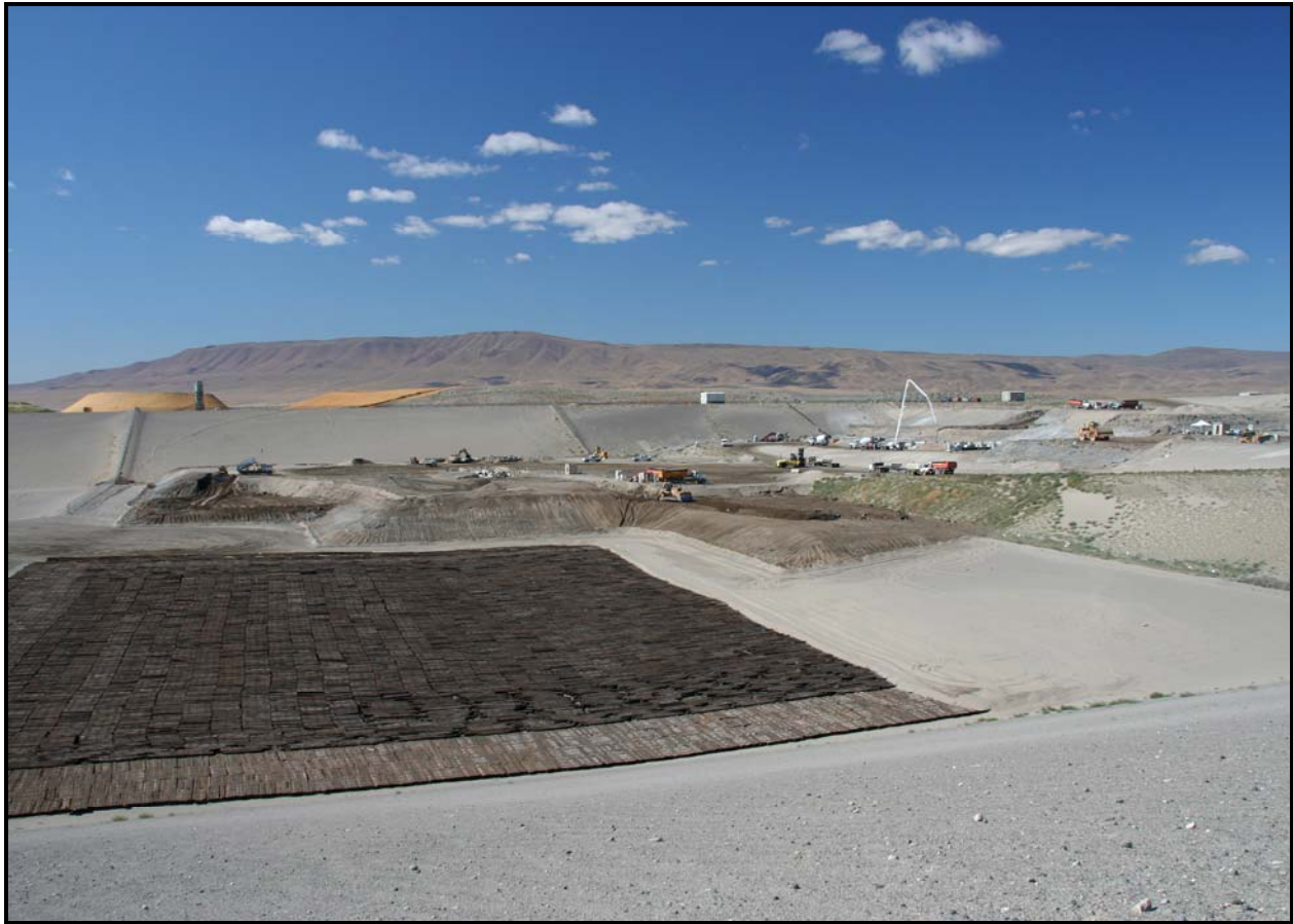
Waste continues to fill super cell 9 at the Environmental Restoration Disposal Facility. Approximately 58,500 rail ties from the Hanford Site cover a large portion of the cell's north side. (Photo 1)
