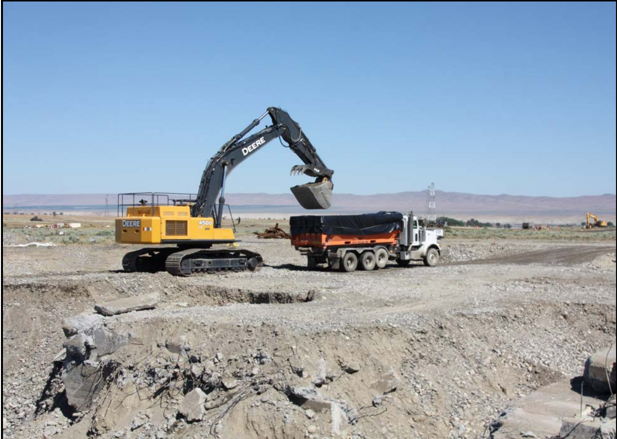
Washington Closure Hanford subcontractor Ojeda Business Ventures continues to load out concrete and soil from 100-F-57. (Photo 7)
