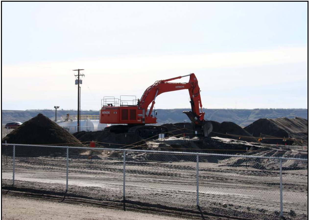
Trench remediation activities continue at the 618-10 Burial Ground. An excavator removes overburden from the northeast corner of the burial ground. (Photo 4)
