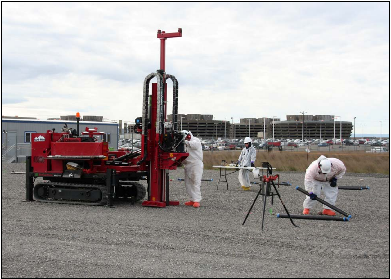
Washington Closure Hanford subcontractor North Wind Inc. began installing cone penetrometers at the 618-11 Burial Ground. The site is located next to the Columbia Generating Station. (Photo 6)
