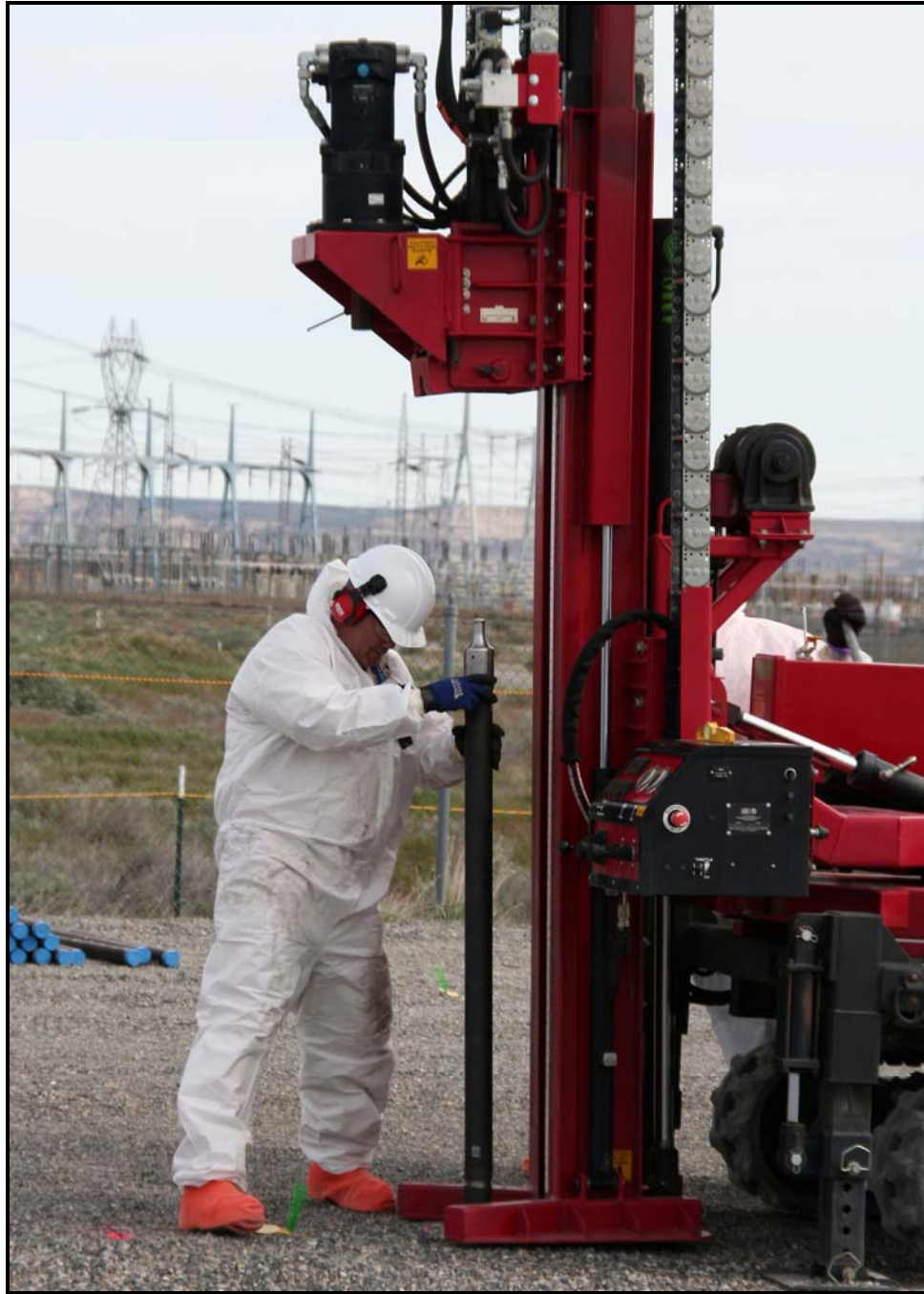
Cone penetrometers are installed to a depth of 6 feet below each vertical pipe unit. (Photo 8)
