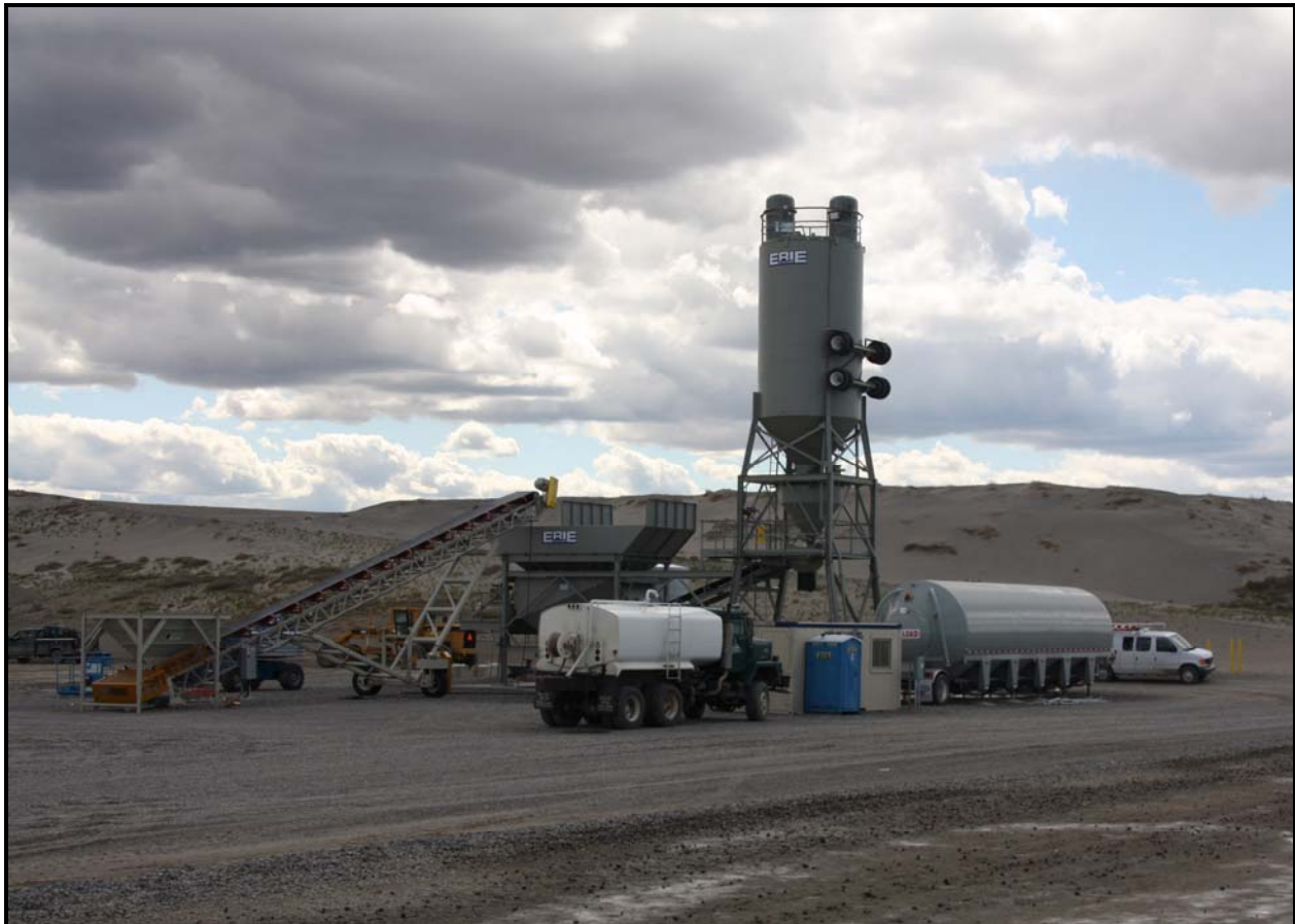
Washington Closure Hanford subcontractor DelHur Industries has completed installation of ERDF's new batch plant. The batch plant is expected to be placed into service in May. (Photo 3)
