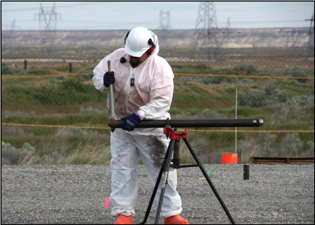
A North Wind Inc. employee prepares a cone penetrometer for installation at the 618-11 Burial Ground. (Photo 7)
