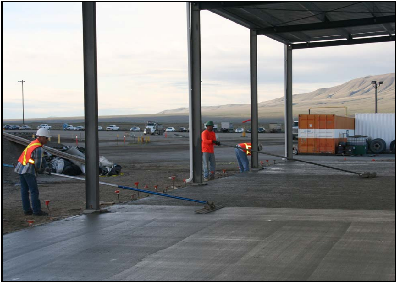
Washington Closure Hanford subcontractor ELRFowler poured another section of concrete for the east addition of ERDF's transportation maintenance facility. (Photo 3)
