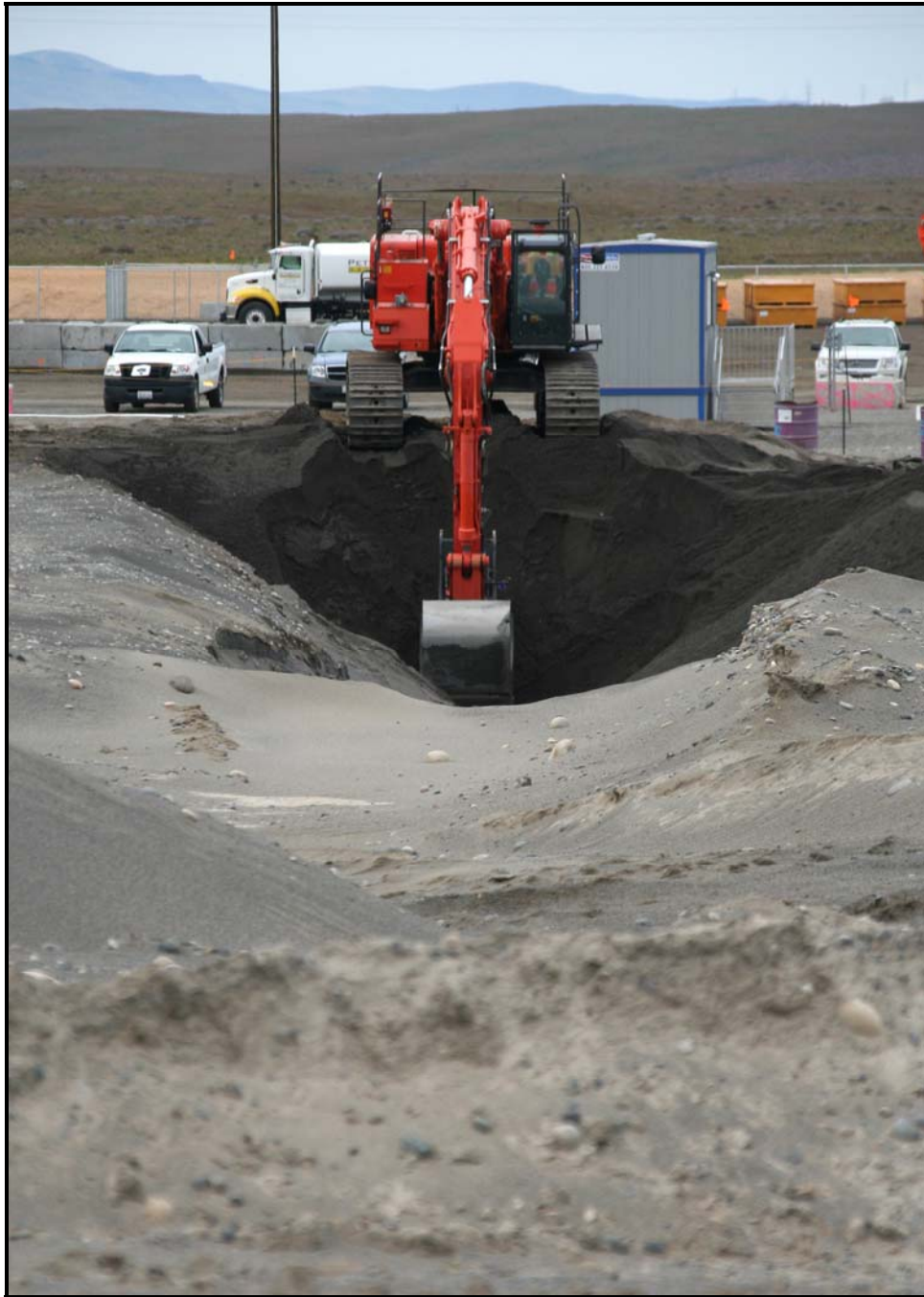
An excavator operator performs mockup exercises at the 618-10 Burial Ground. Remediation of the burial ground's trenches is scheduled to begin next week. (Photo 5)
