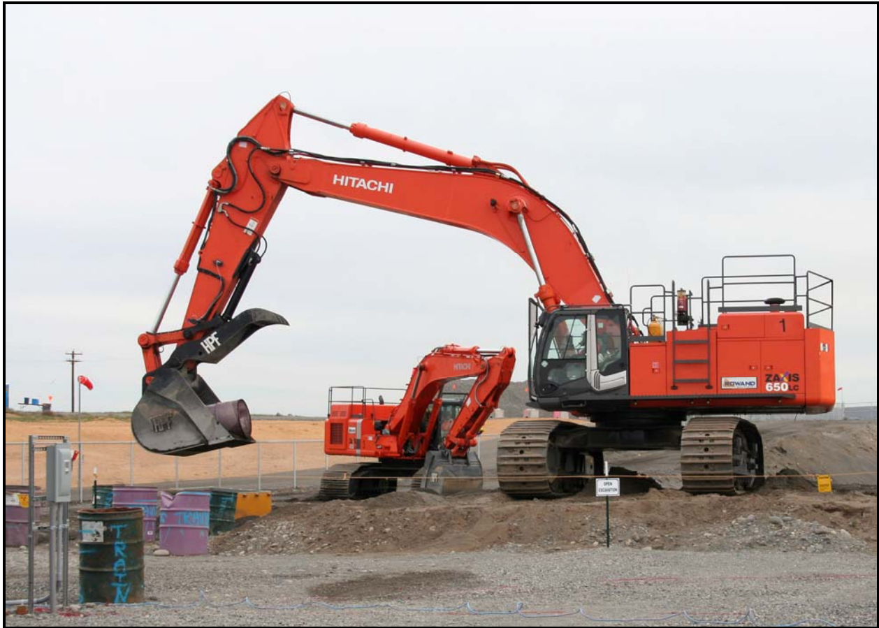
An excavator operator prepares to place a drum into a salvage container during mockup exercises at the 618-10 Burial Ground. (Photo 6)
