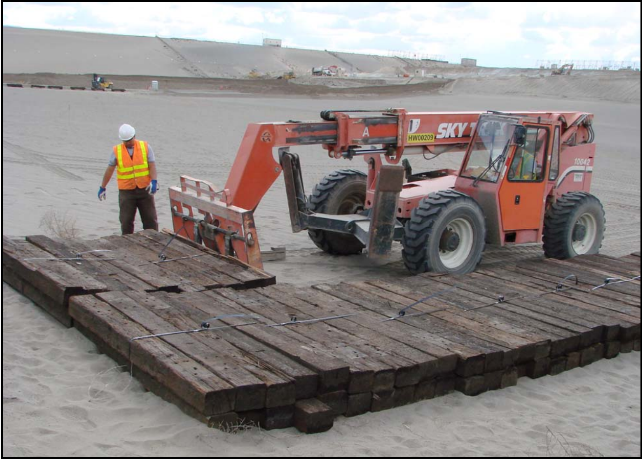
ERDF personnel began disposing of contaminated railroad ties in super cell 9. The construction of super cell 9 is part of a $100 million expansion and upgrade of the facility. (Photo 2)
