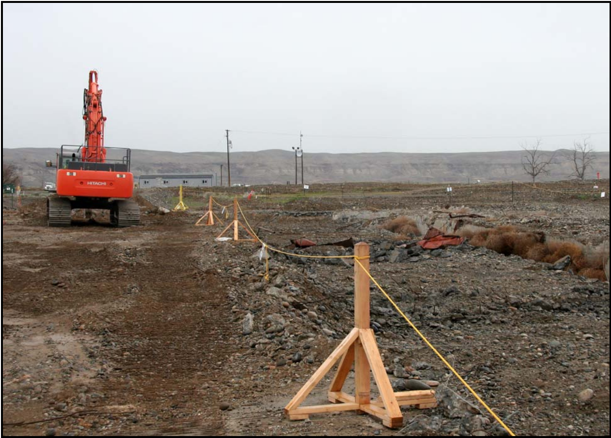
Waste site 100-F-57 was found to contain stained concrete and soil containing hexavalent chromium. (Photo 9)
