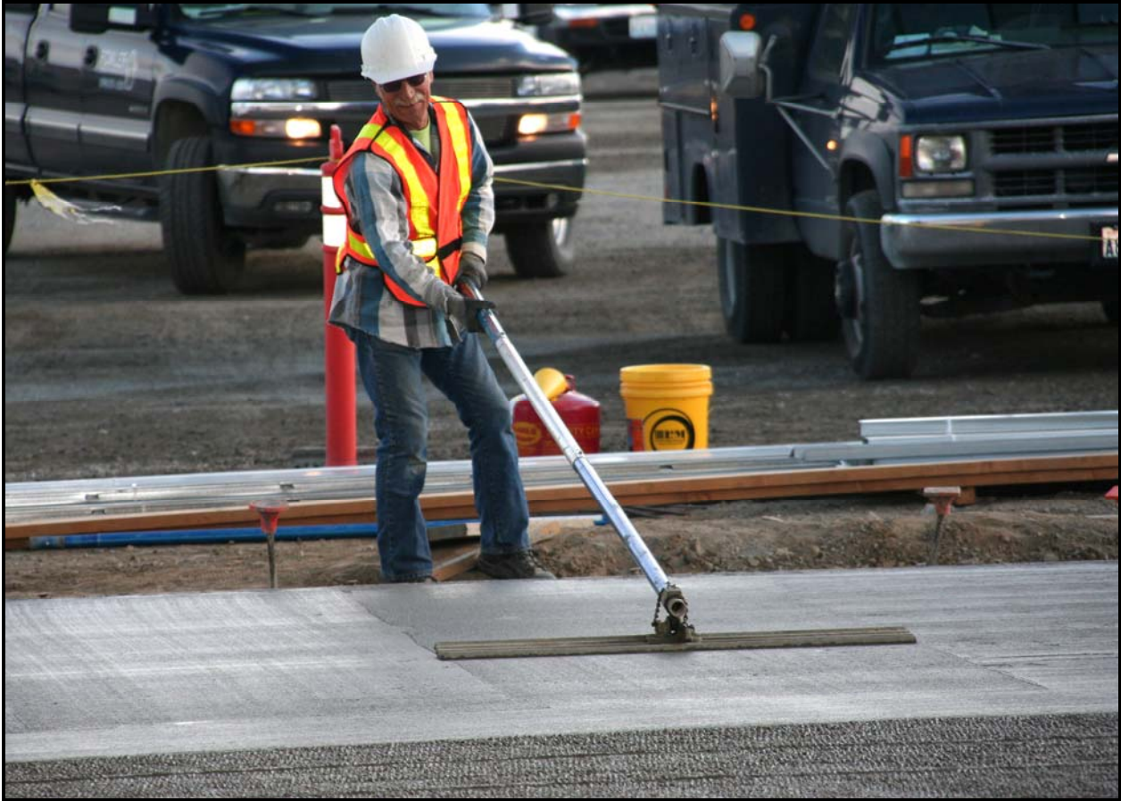
An ELRFowler employee floats a section of the recently poured concrete slab for the east addition of the container maintenance facility. (Photo 4)
