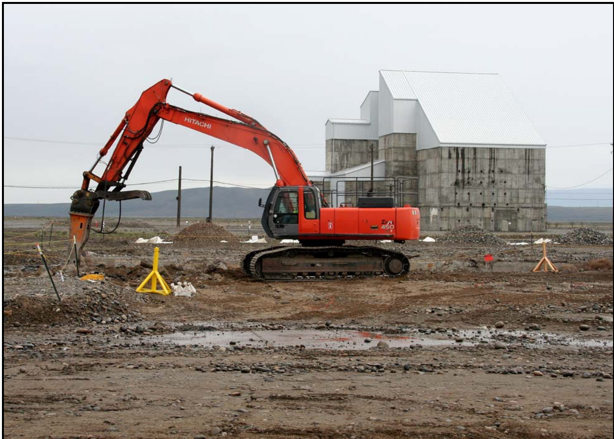
Washington Closure Hanford subcontractor Ojeda Business Ventures demolishes concrete slabs at 100-F-57, a waste site located near F Reactor. (Photo 8)
