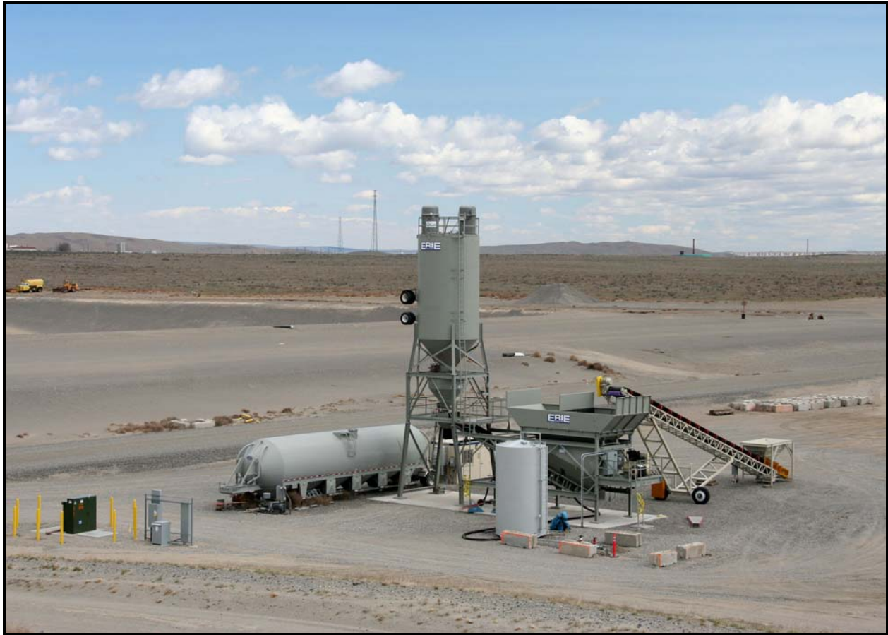
Washington Closure Hanford subcontractor DelHur Industries has installed the conveyer and hopper for ERDF's new batch plant. (Photo 4)
