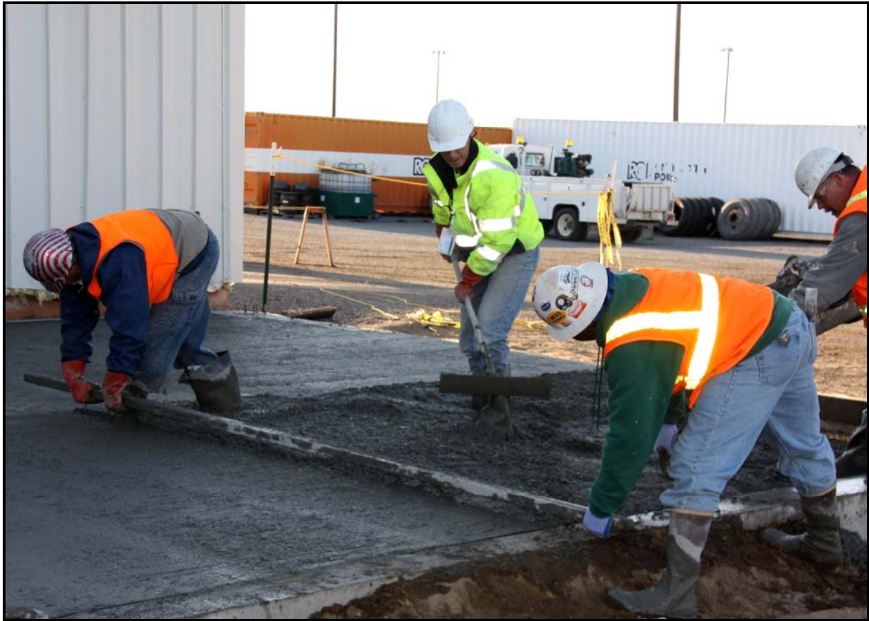
Washington Closure Hanford subcontractor ELRFowler pours the concrete slab for the west addition of ERDF's transportation maintenance facility. (Photo 1)
