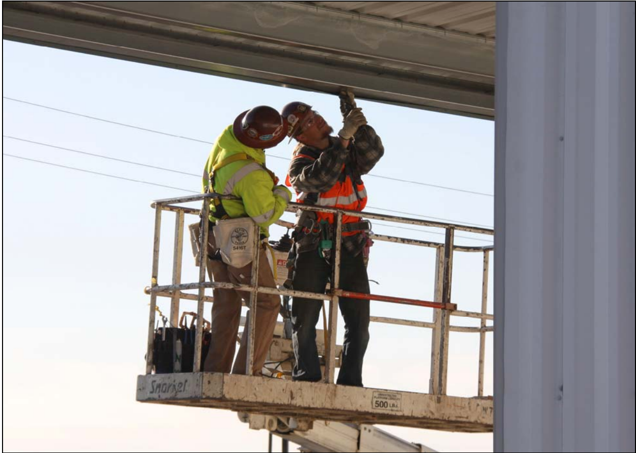
ELRFowler employees work on an awning at ERDF's transportation maintenance facility. (Photo 3)
