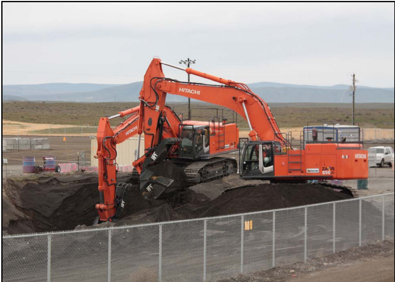
Mockup exercises continue at the 618-10 Burial Ground. Full-scale trench remediation is expected to begin next week. (Photo 5)
