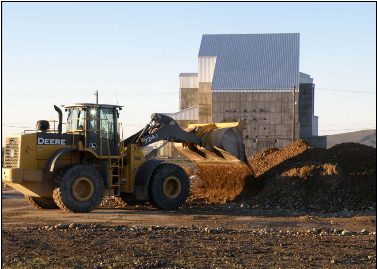
Washington Closure Hanford subcontractor Ojeda Business Ventures removes overburden from 100-F-57. The site contains hexavalent chromium. (Photo 8)
