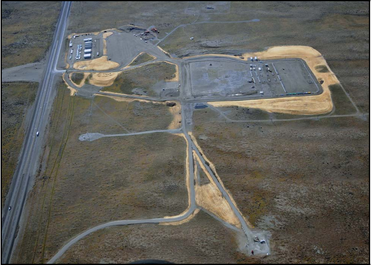
The 618-10 Burial Ground is one of the most complex remediation projects on the Hanford Site. The six-acre burial ground operated from 1954 to 1963. (Photo 6)
