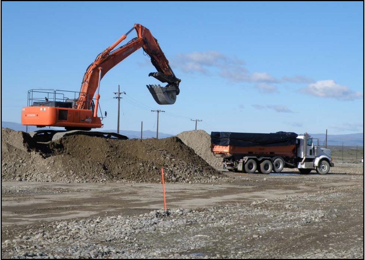
Ojeda removes overburden from 100-F-57. Next week, the project team plans to begin breaking concrete slabs containing hexavalent chromium. (Photo 9)
