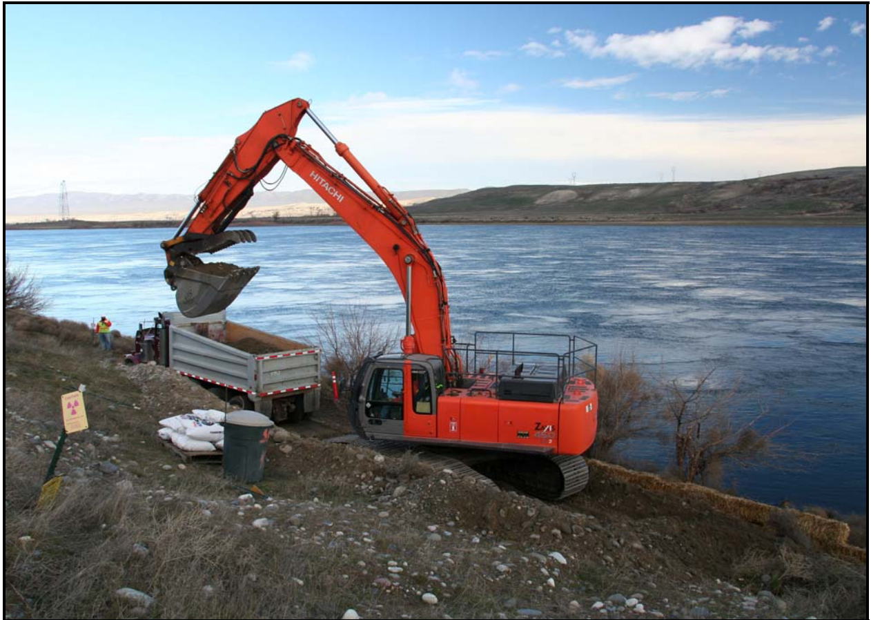
Washington Closure Hanford subcontractor Ojeda Business Ventures begins excavation and loadout at waste site 100-F-45. The site is located on the bank of the Columbia River. (Photo 4)
