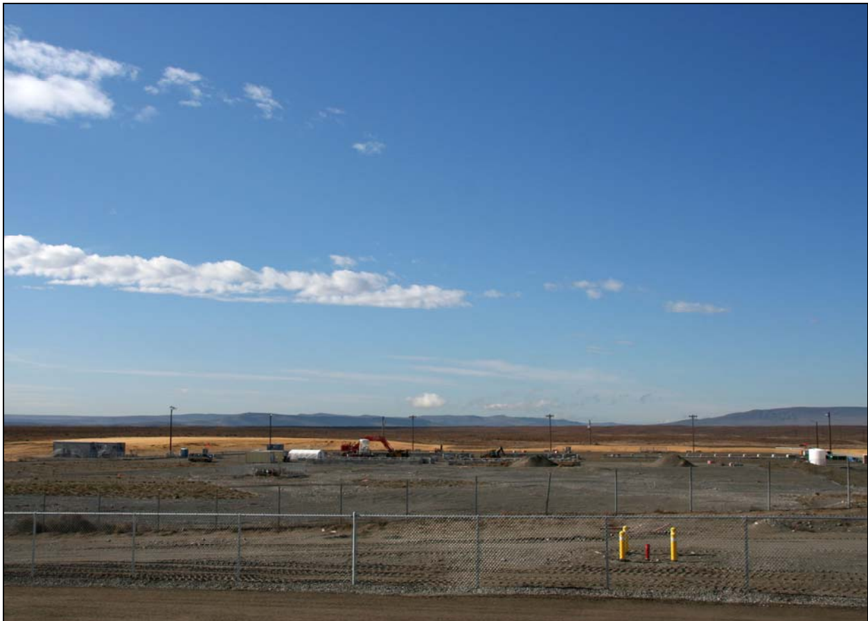
Washington Closure Hanford is preparing to begin excavating surge trenches next week at the 618-10 Burial Ground. (Photo 2)
