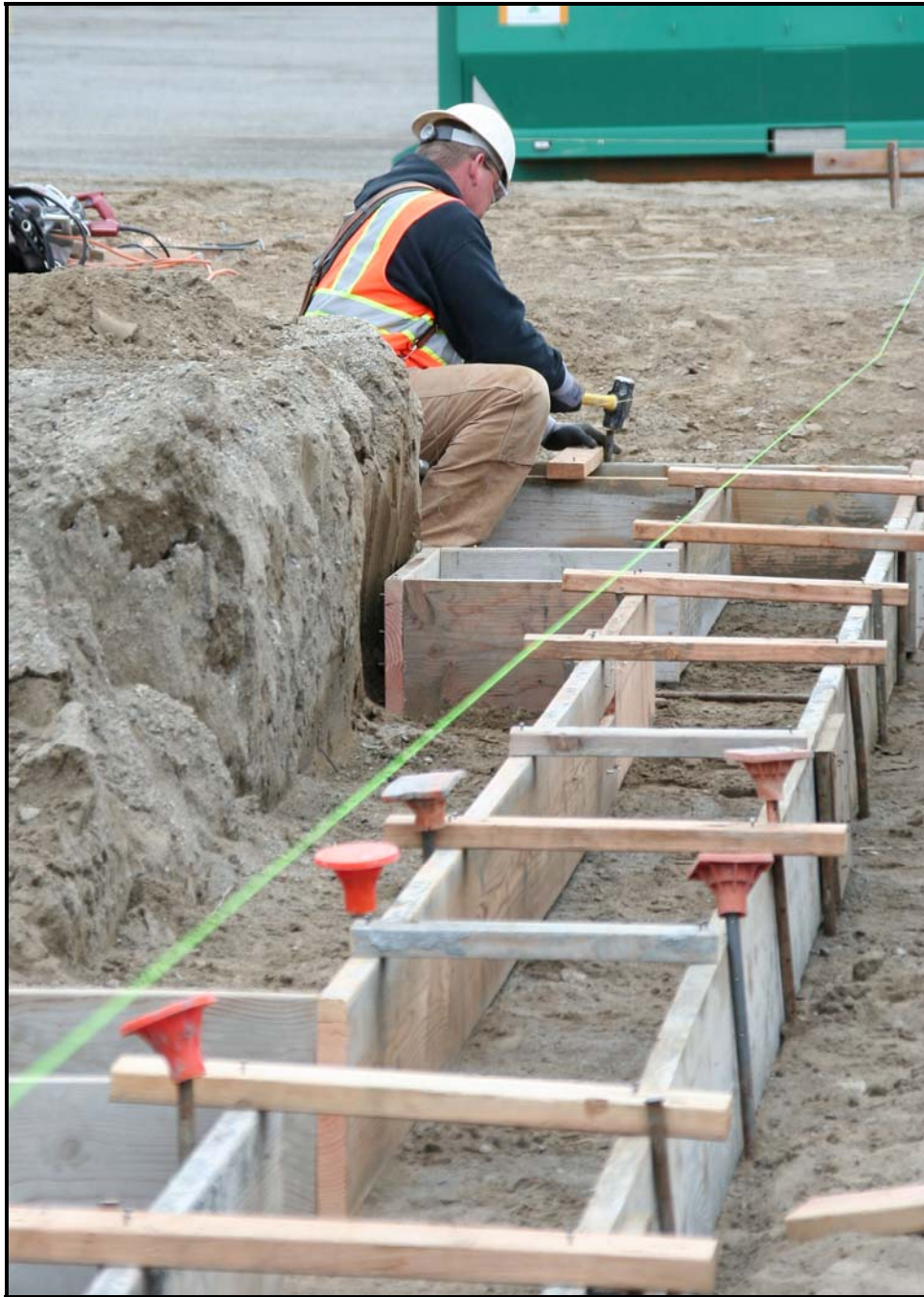
An employee with Washington Closure Hanford subcontractor ELRFowler constructs forms used to pour concrete footers at the transportation maintenance facility. (Photo 1)
