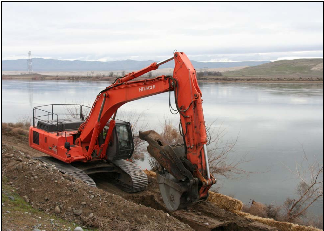
An excavator scoops out a section of river outfall pipeline at 100-F-45. The pipeline was used to discharge effluent into the Columbia River. (Photo 5)
