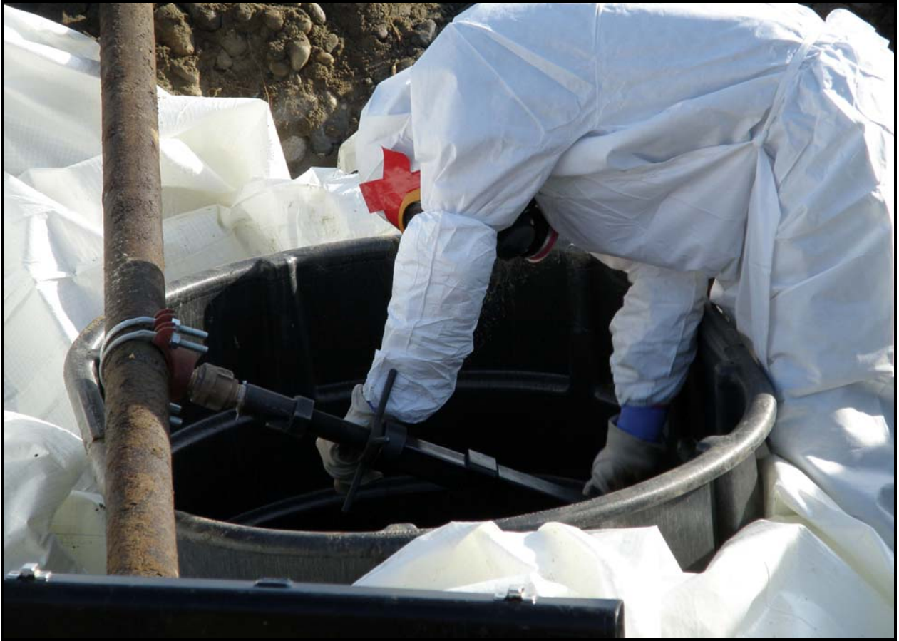
Washington Closure Hanford subcontractor Ojeda Business Ventures drains liquid from a pipe at 100-F-26:7. The site contains sodium dichromate and sodium silicate pipelines. (Photo 8)
