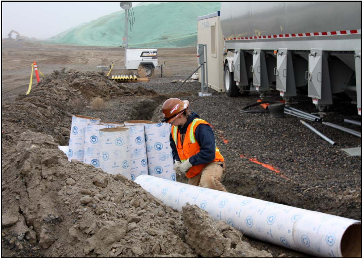
Electrical work continues for the new batch plant at the Environmental Restoration Disposal Facility. (Photo 3)
