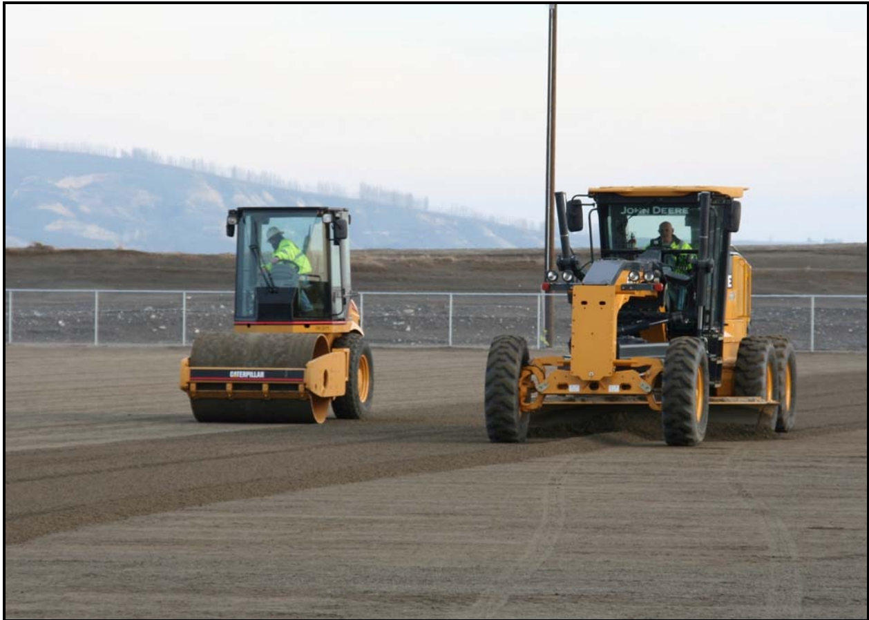
Washington Closure Hanford subcontractor White Shield/Apollo grades the staging area at the 618-10 Burial Ground. (Photo 4)
