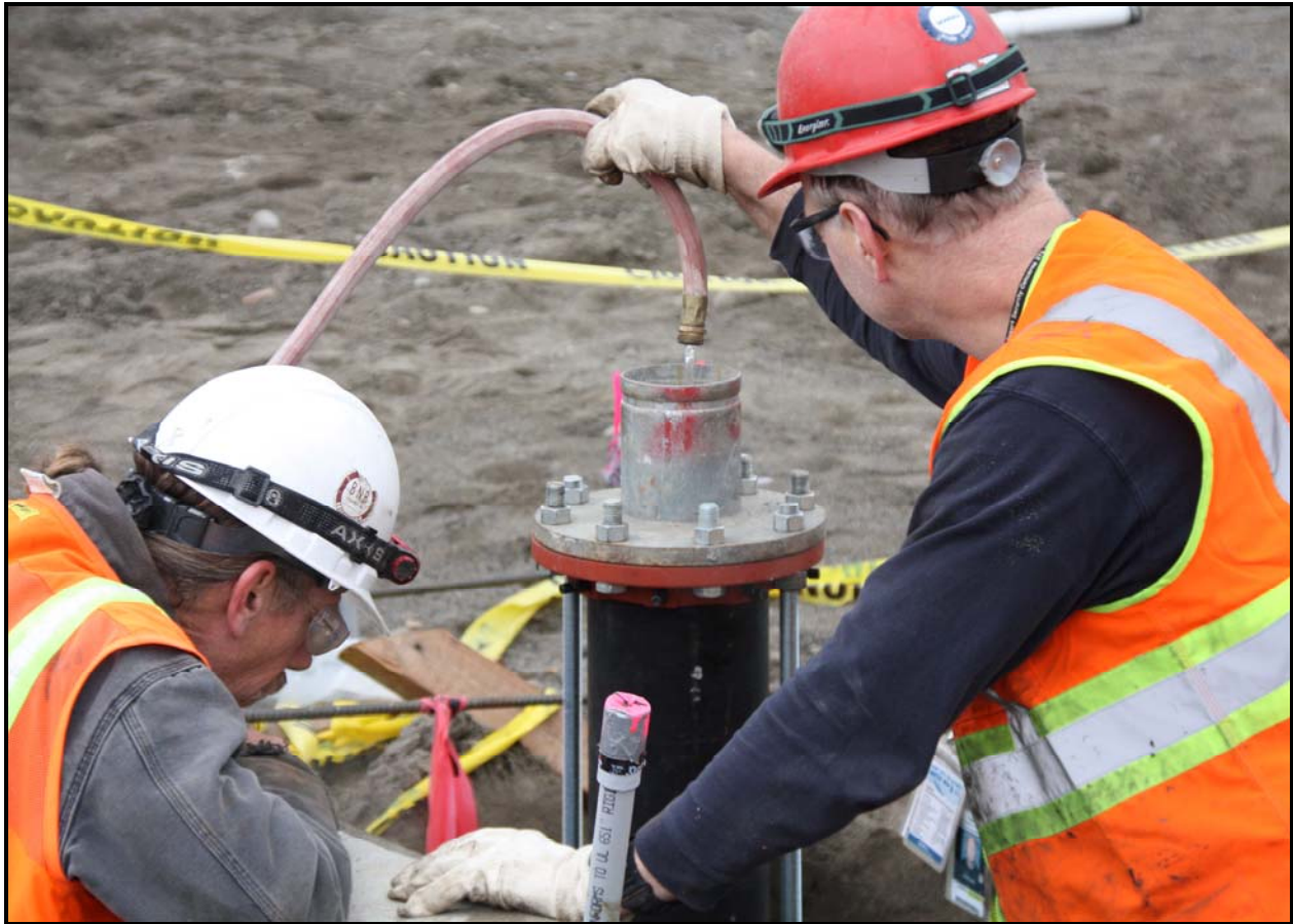
ELRFowler employees conduct a hydrostatic test on a fire riser at the equipment maintenance facility/operations center. (Photo 2)
