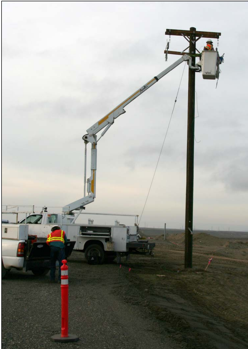
Workers continue to install light polls along site roads at the 618-10 Burial Ground. (Photo 5)
