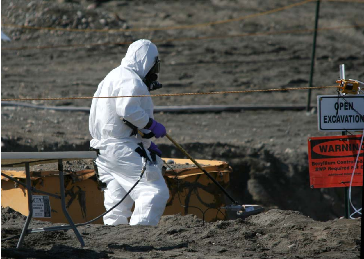
A radiological control technician takes a reading during trench excavation at the 618-10 Burial Ground. (Photo 8)
