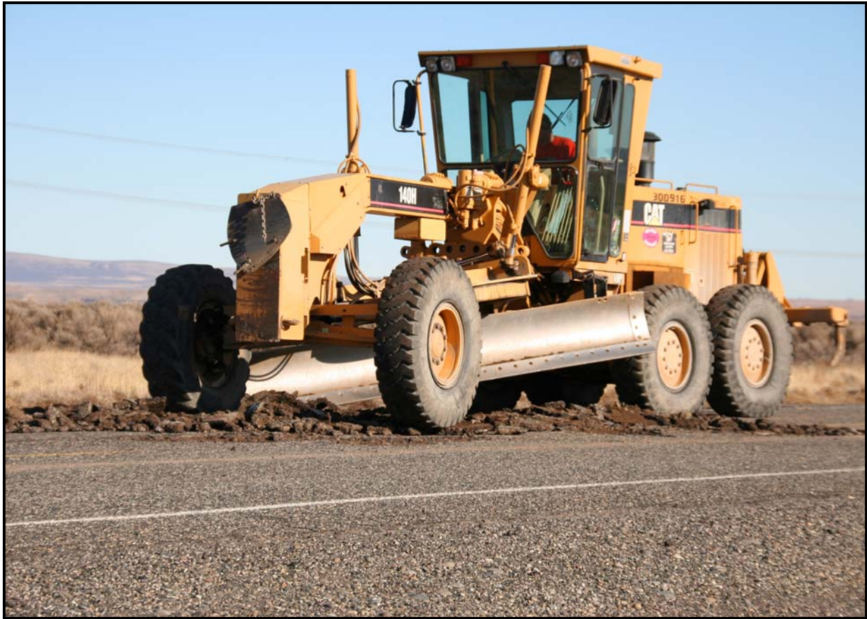
Road crews begin to scrape a 900-foot section of Route 1 that will require a 2-inch overlay of asphalt.
