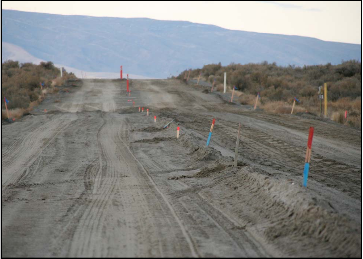
George A. Grant Inc. completed subgrading the back road to ERDF and is scheduled to begin paving November 30.
