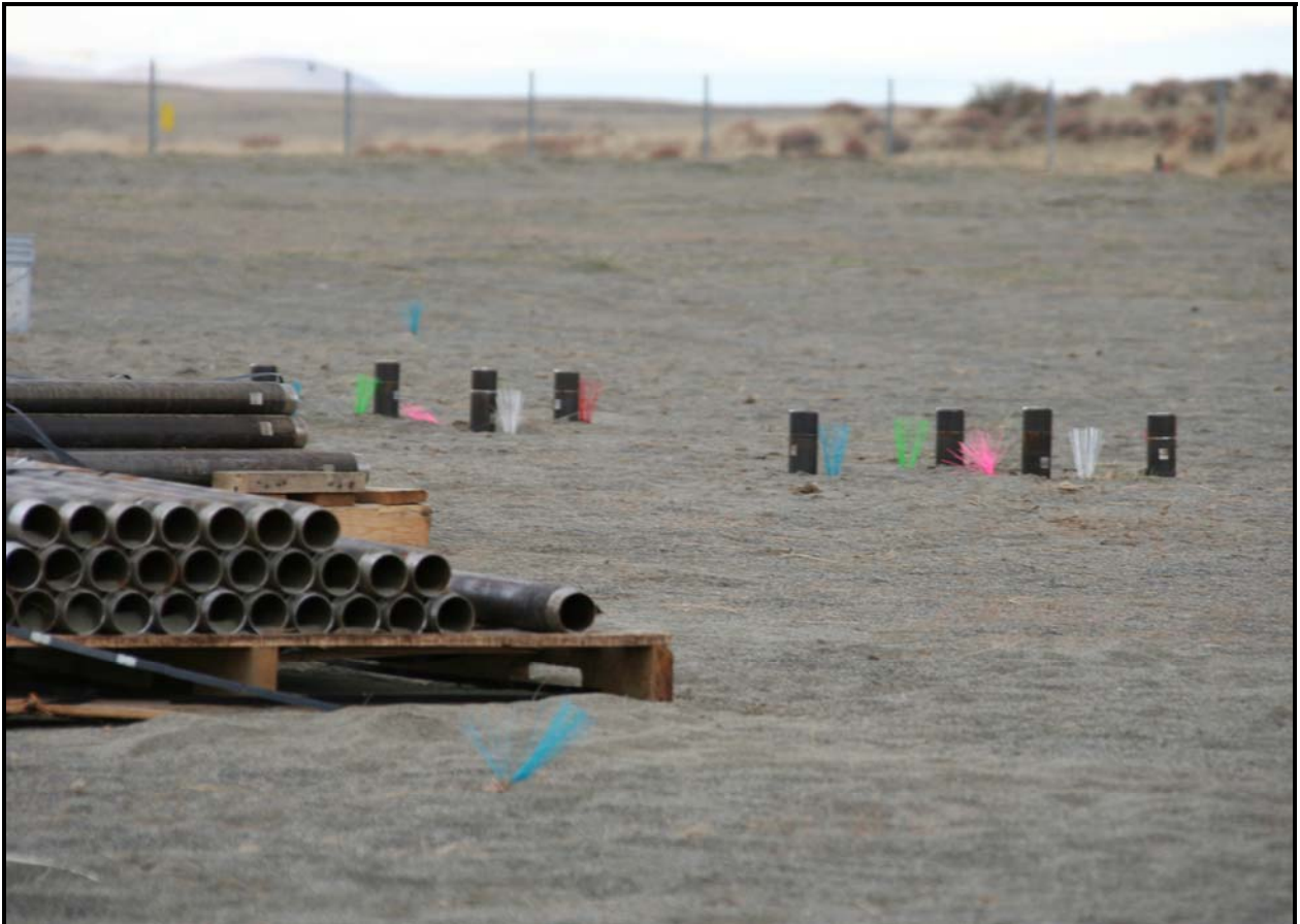
North Wind Inc. has installed 236 cone penetrometers to a depth of 8 feet at the 618-10 Burial Ground.
