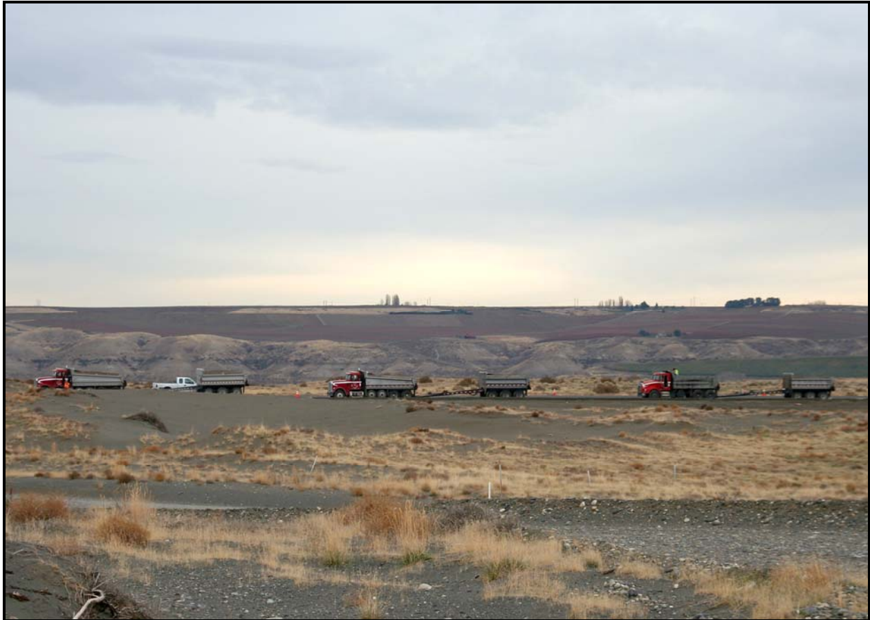
Road crews completed paving the median and the entrance/exit lanes at the 618-10 Burial Ground.
