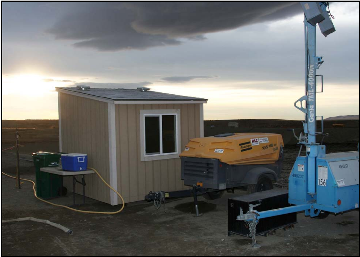
A ramp shack was installed at the Environmental Restoration Disposal Facility. The shack provides a place to store tools and equipment, and to process paperwork.
