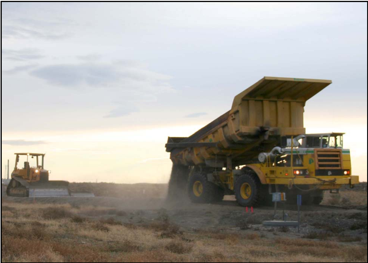
Fill dirt is dumped on the back road into the Environmental Restoration Disposal Facility.
