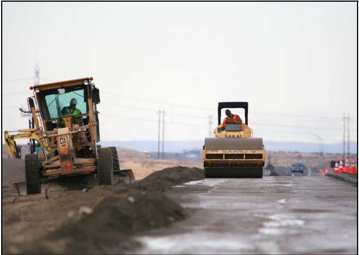
Road crews continue to prepare the entrance/exit lanes for paving at the 618-10 Burial Ground.
