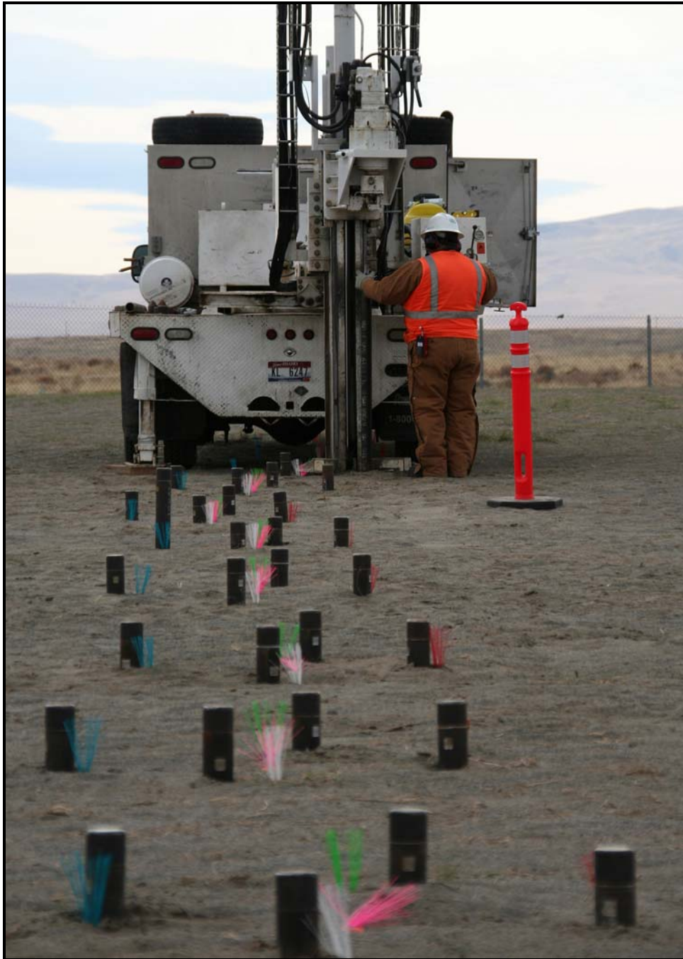
North Wind Inc. workers continue to install cone penetrometers around the vertical pipe units at the 618-10 Burial Ground.
