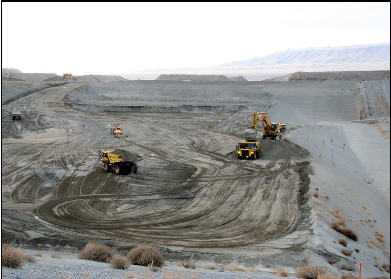
DelHur Industries continues excavation at super cell 9. Excavation work is about 60 percent complete.
