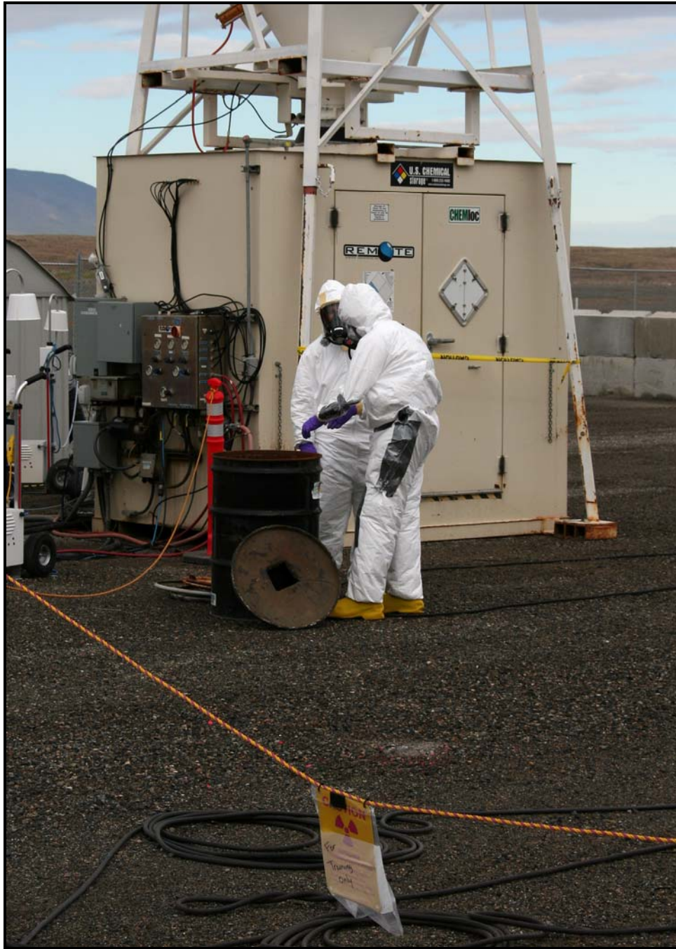
The project team at the 618-10 Burial Ground is scheduled to conduct mock-ups of the drum punch facility next week.
