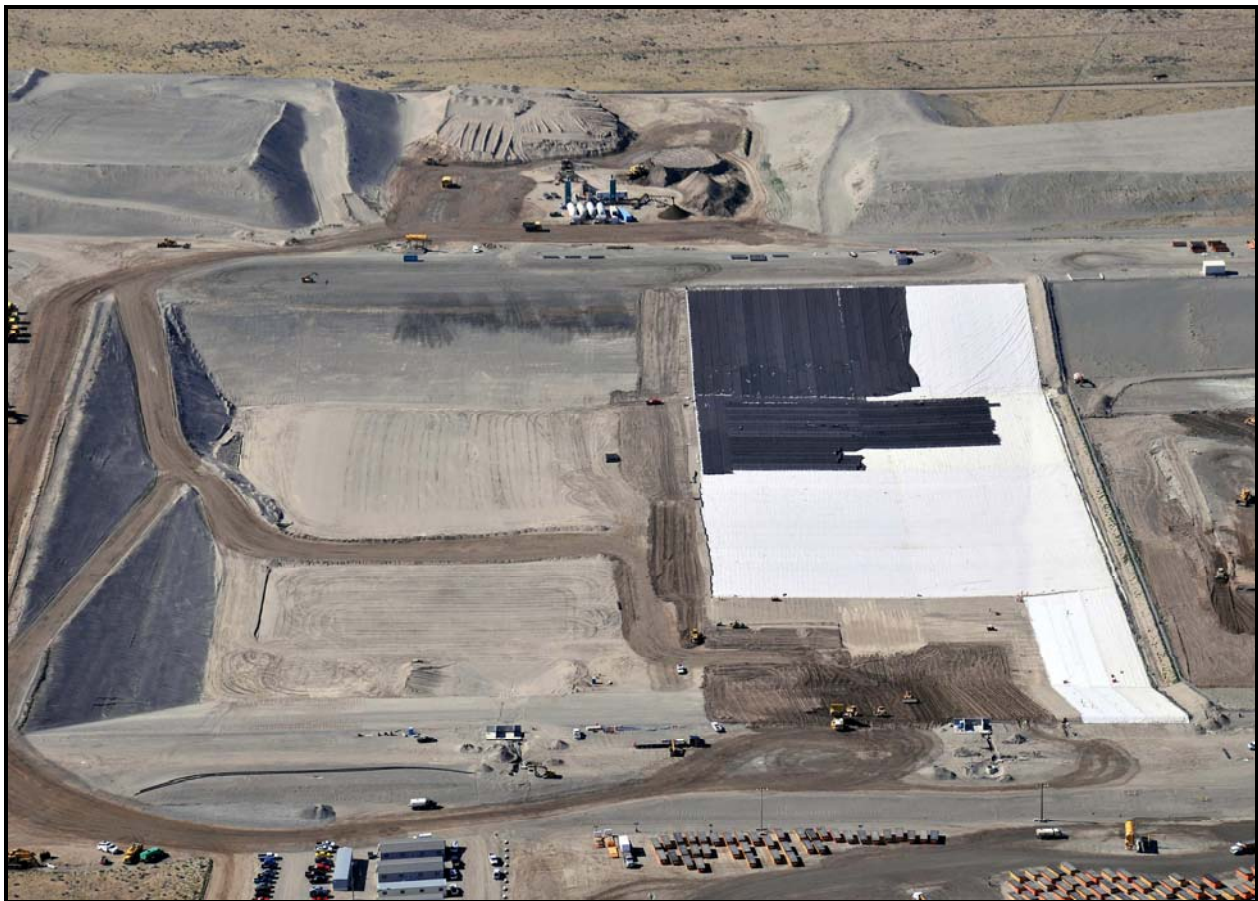
An aerial photo was taken June 29 from the north side of super cells 9 and 10 at the Environmental Restoration Disposal Facility.
