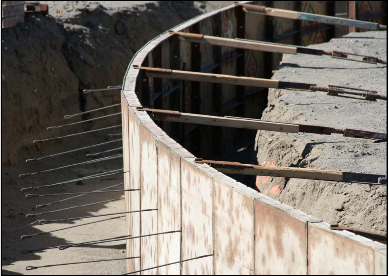
Construction of a new leachate holding tank continues at the Environmental Restoration Disposal Facility. The tank will accommodate leachate from super cells 9 and 10.
