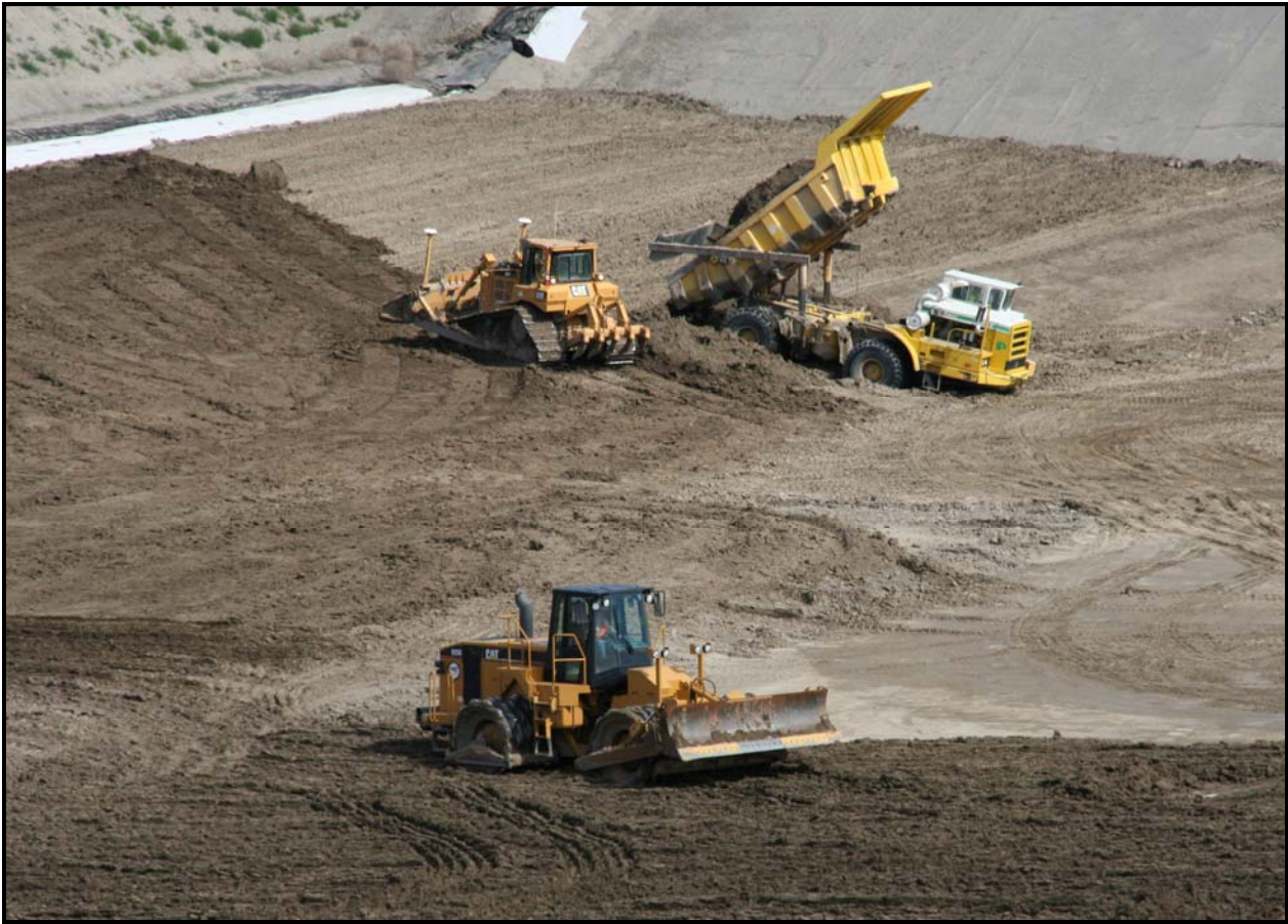
TradeWind Services/DelHur Industries personnel continue to place admix in super cell 9 at the Environmental Restoration Disposal Facility. About 50% of the admix layer has been placed.
