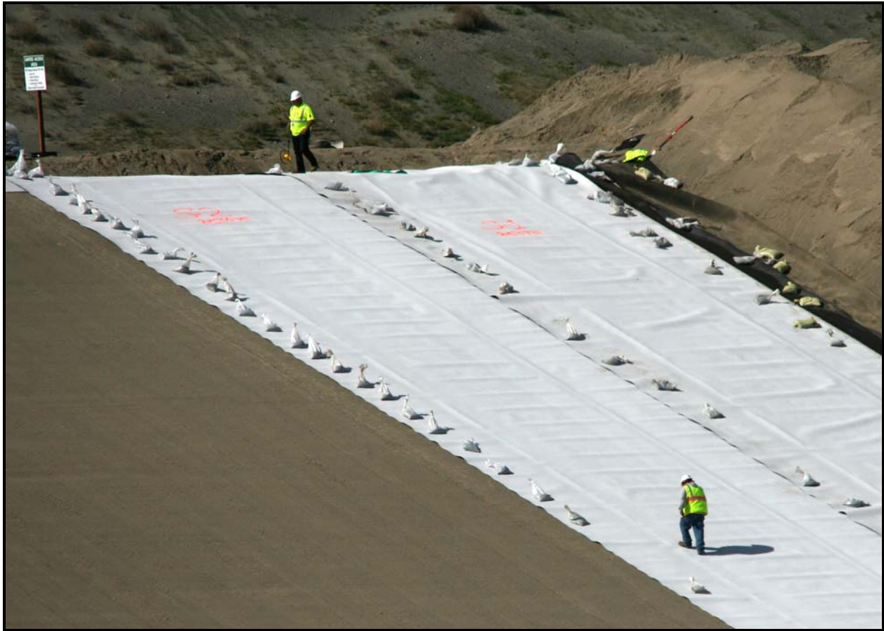
Each roll of HDPE measures 540-feet long by 22-feet wide. The rolls are heat welded together to cover the super cell, which measures 500 feet by 1,000 feet at the base.
