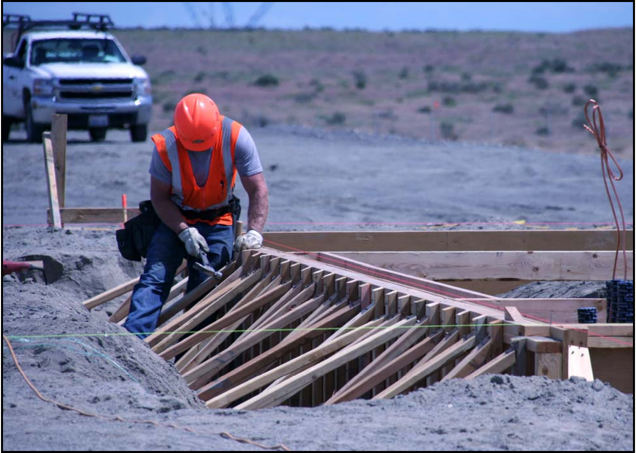
Work continues on the foundation for the super cell 10 crest pad building at the Environmental Restoration Disposal Facility.
