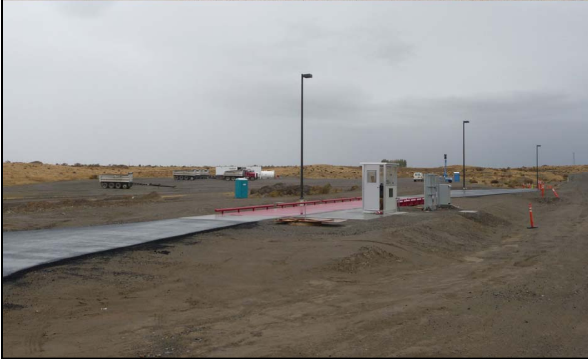
Work began on the third scale in September (top). As of October 25 aprons had been added to the scale (bottom).
