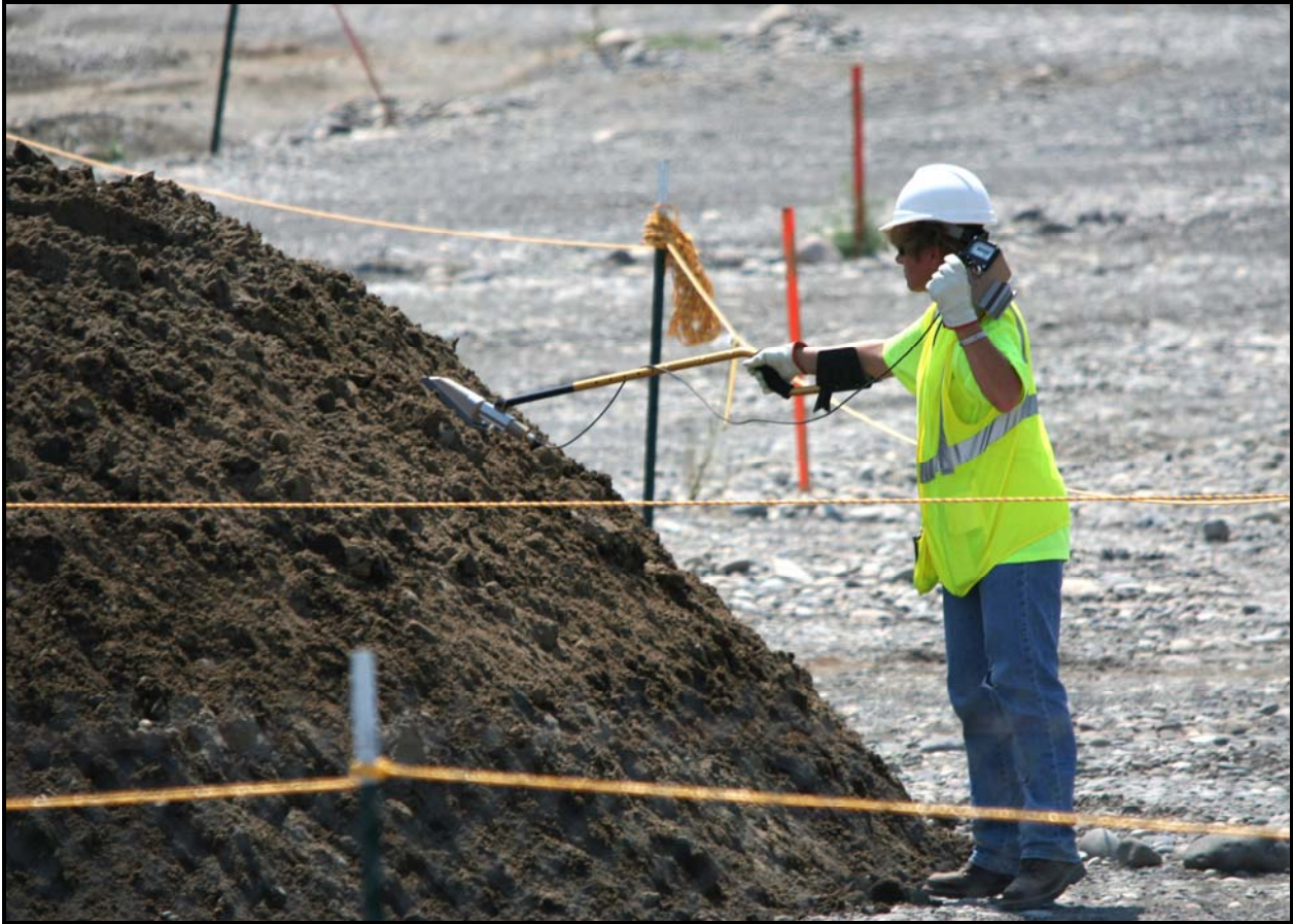
A radiological control technician takes a measurement of soil after excavation of a surge pit at the 618-10 Burial Ground.
