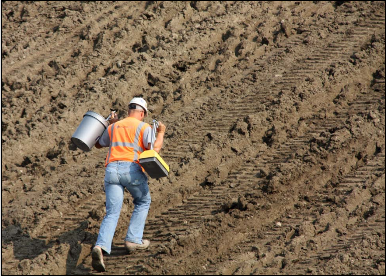
An employee from Envirotech prepares to test the compaction of admix on the north slope of super cell 10 at the Environmental Restoration Disposal Facility.
