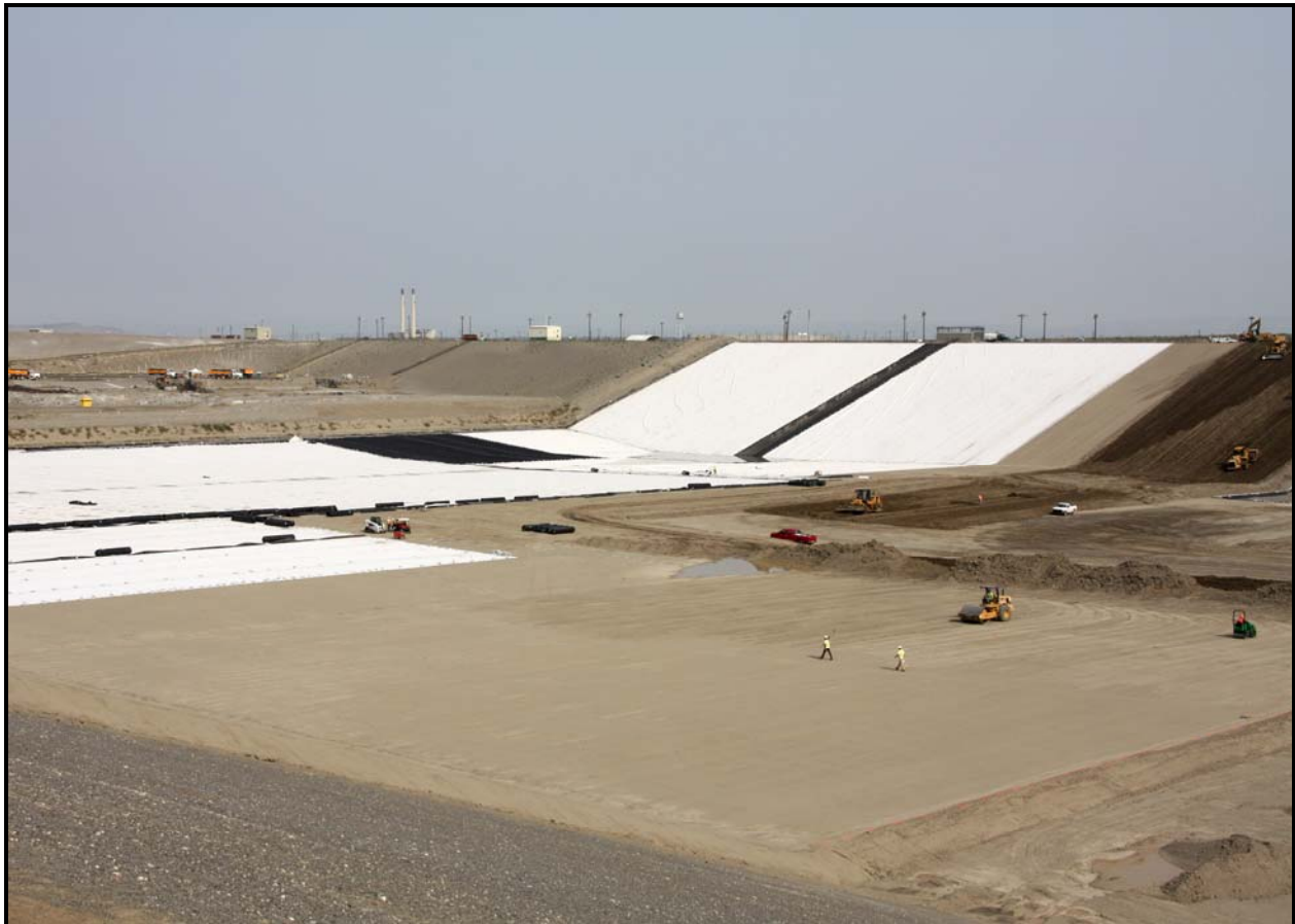
A photograph from the southeast corner of super cell 10 shows liner construction at the Environmental Restoration Disposal Facility.
