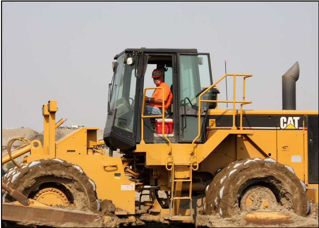
A TradeWind Services/DelHur Industries employee runs a sheepfoot compactor during admix placement in super cell 10 at the Environmental Restoration Disposal Facility.
