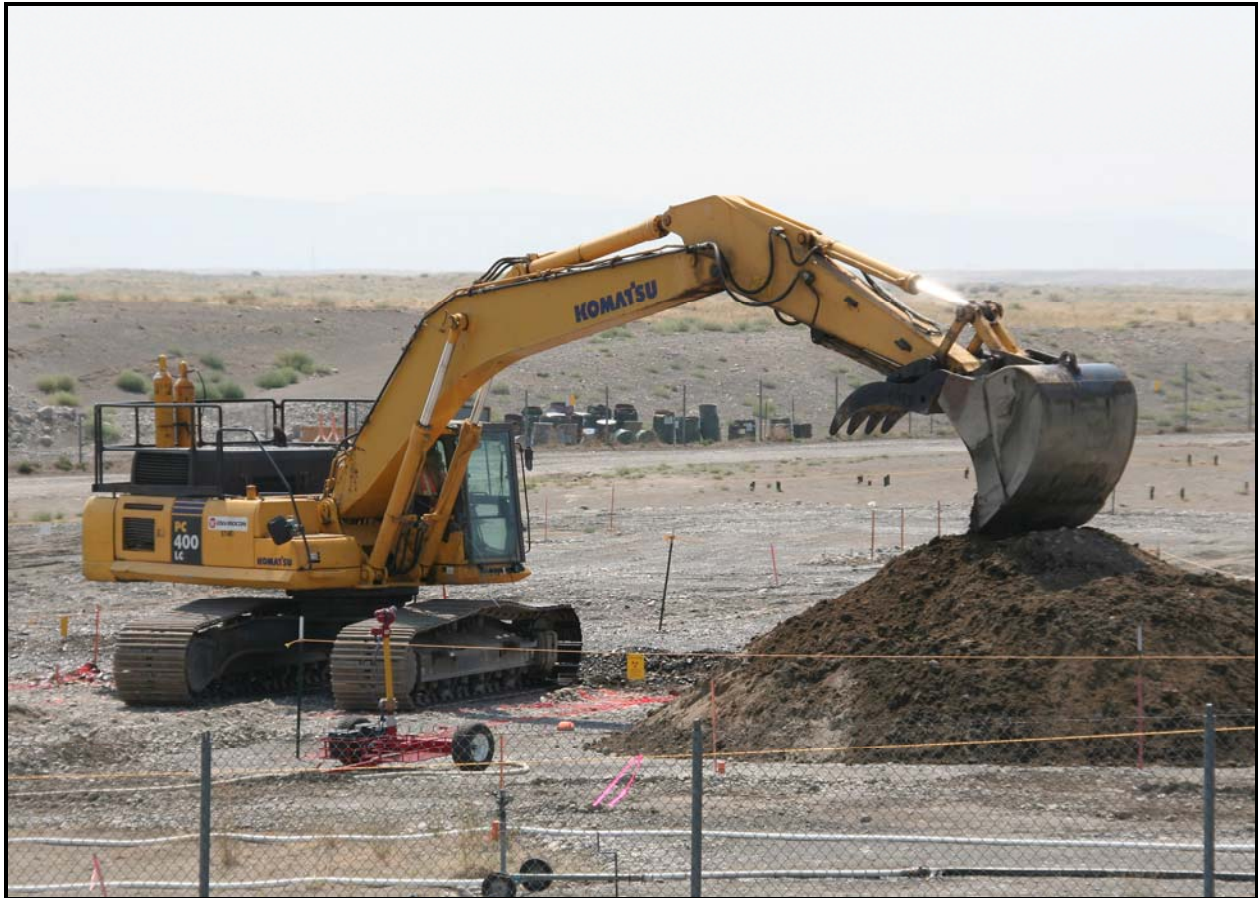
A track-hoe excavates a surge trench as intrusive characterization field operations began at the 618-10 Burial Ground.
