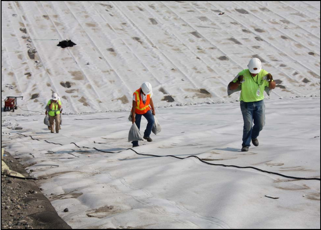
Environmental Services Inc. employees carry sandbags up the south slope of super cell 9 during the installation of the liner system at the Environmental Restoration Disposal Facility.
