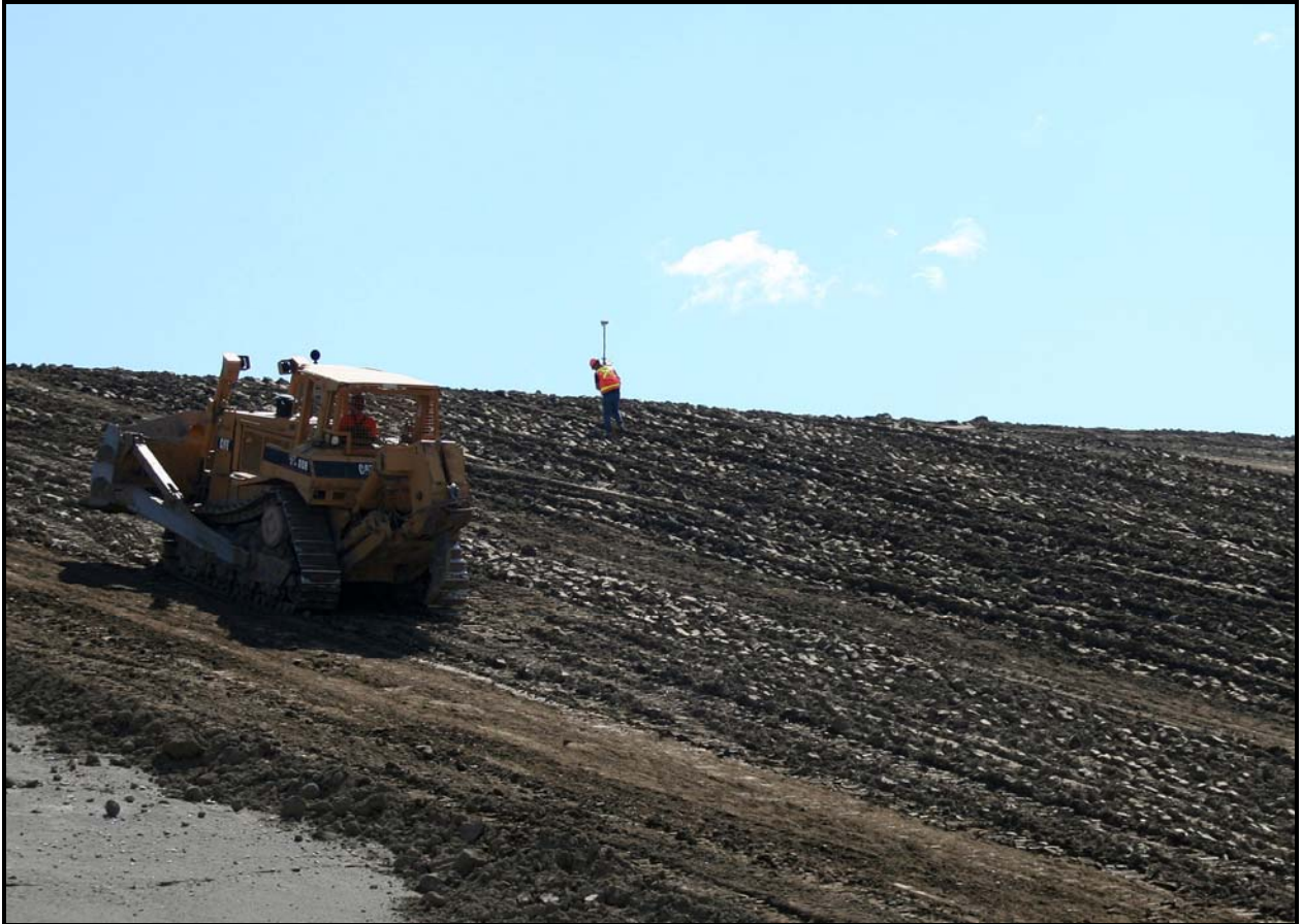
Work crews place admix on the south slope of super cell 9 at the Environmental Restoration Disposal Facility.
