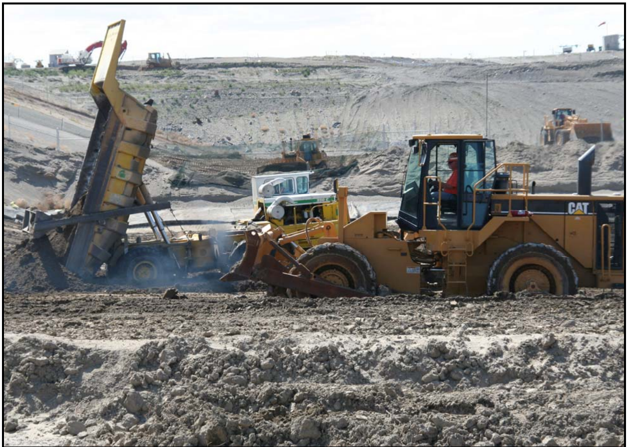
TradeWind Services/DelHur Industries personnel begin placing admix in super cell 9 at the Environmental Restoration Disposal Facility. The admix is used for the compacted soil liner of the liner and leachate collection system.
