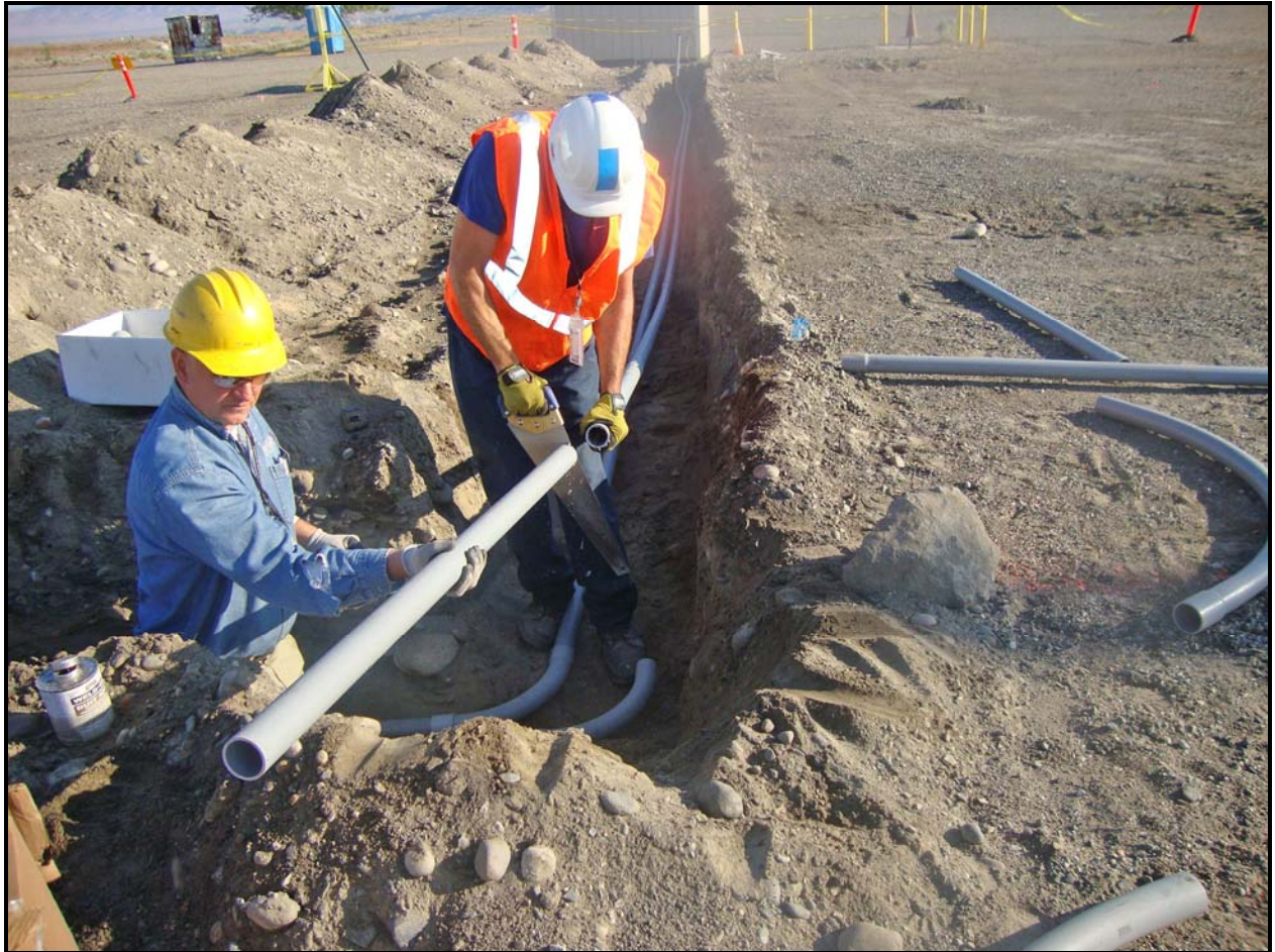
Work to install electrical conduit at 100-F Area continues in preparation of remediation activities.
