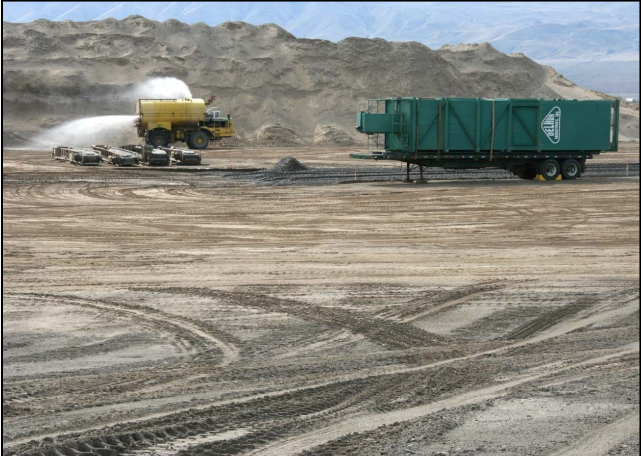
DelHur Industries prepares the pug mill site at the Environmental Restoration Disposal Facility.
