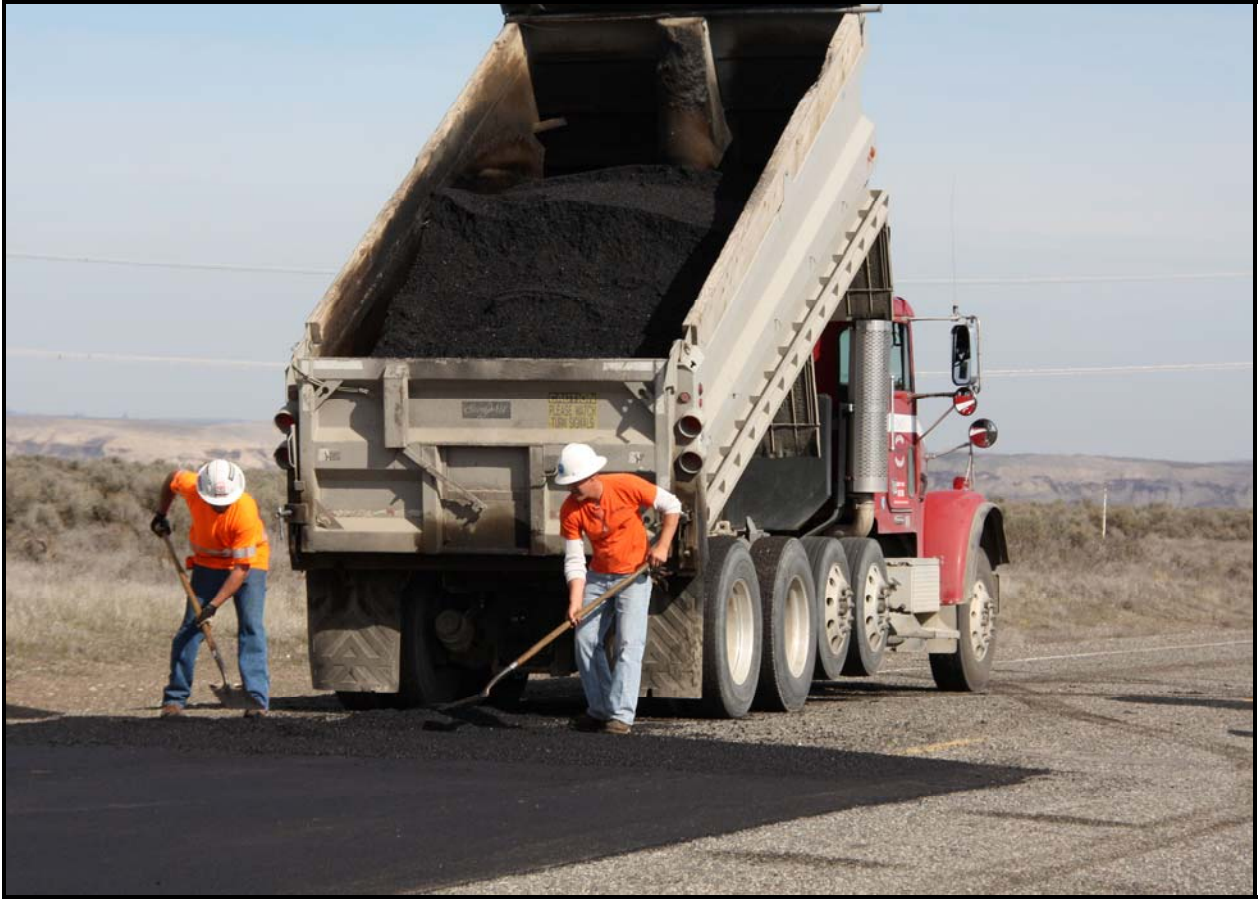
Workers from Inland Asphalt Company pave a problem area on Route 1 at the Hanford Site.
