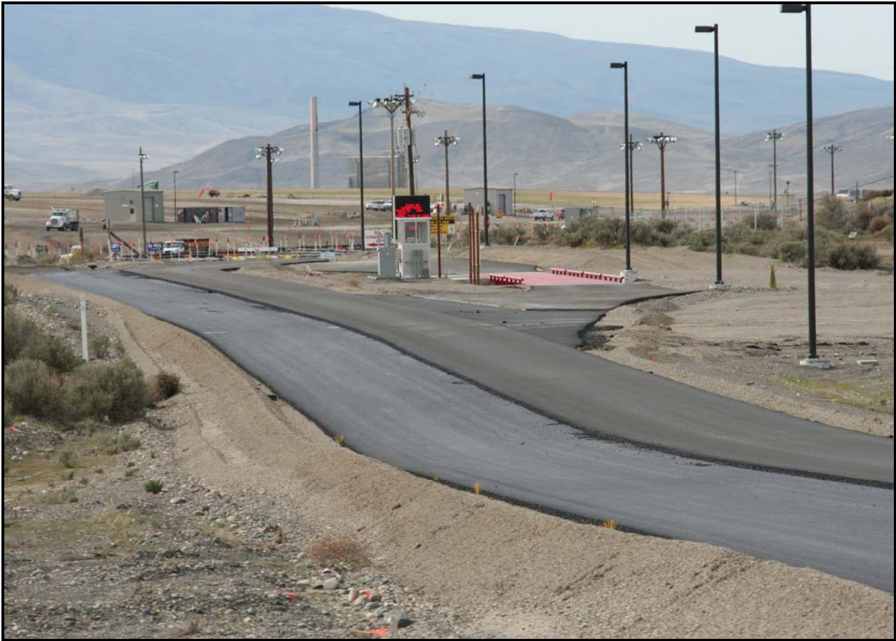
Inland Asphalt Company completed paving the back road to the Environmental Restoration Disposal Facility. The new scale is operational.
