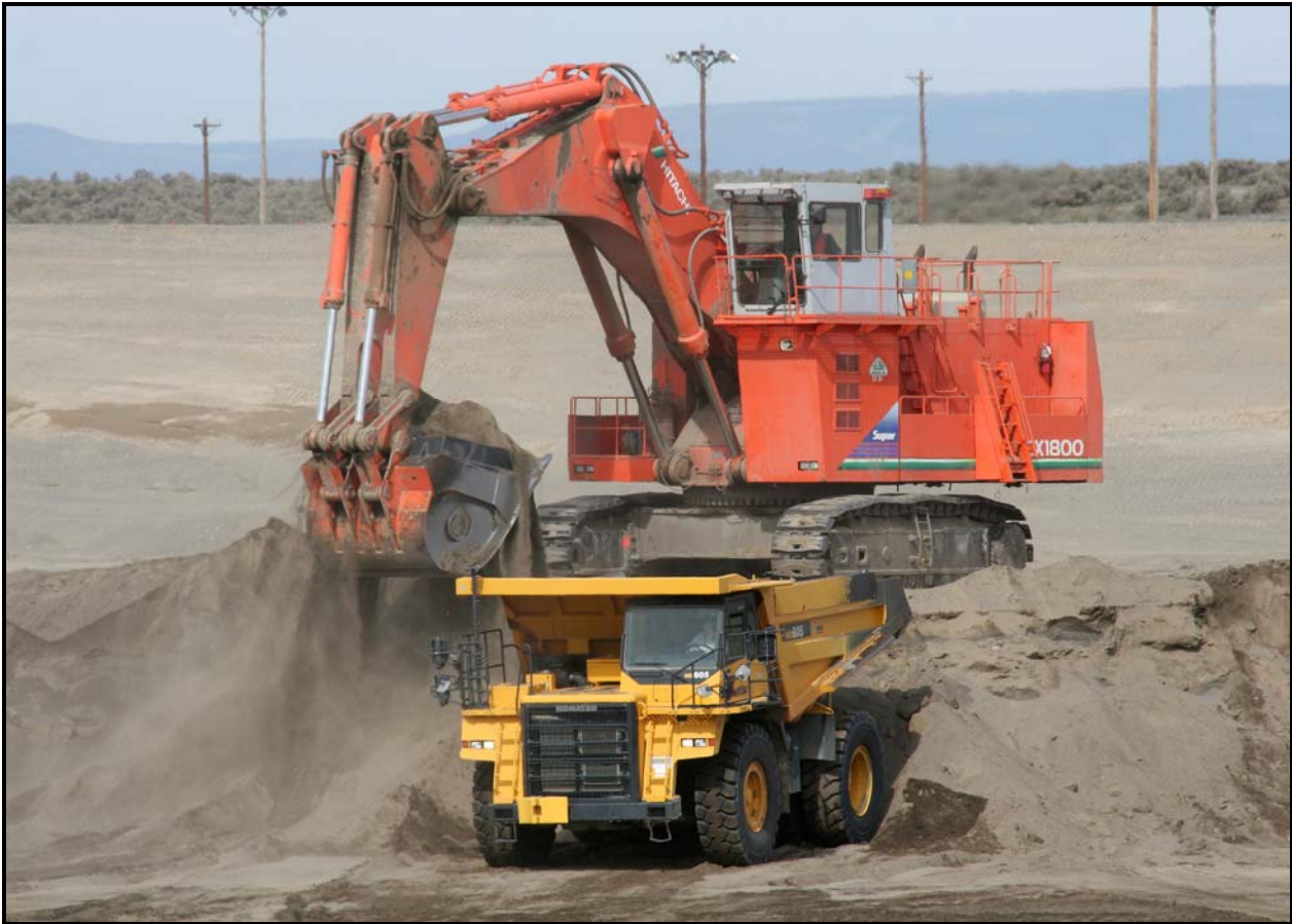
Work continues with the preparatory work of super cell 10 at the Environmental Restoration Disposal Facility.
