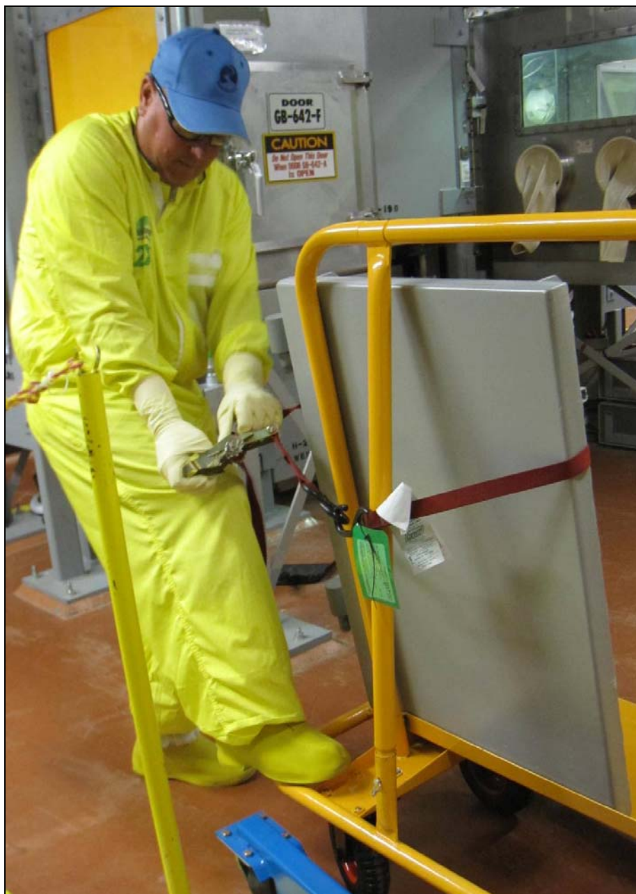
A nuclear chemical operator secures shielding from a glove box in the 2736-Z/ZB facility for removal from the room. Removal of the shielding is necessary to allow for cleanout and size reduction of the glove box.
