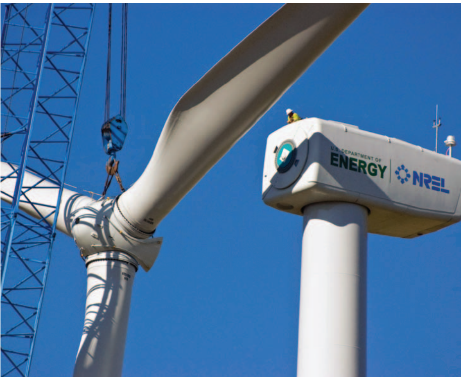
National Renewable Energy Laboratory technicians install DOE's 1.5-megawatt GE wind turbine at the National Wind Technology Center. Photo by Pat Corkery, NREL/PIX 16571
