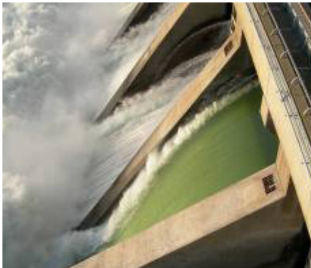
Fish weir slide gives safer ride: The smooth green water of a fish weir (closest spillway) lets young salmon slide over a dam in the surface water they prefer. (Photo: U.S. Army Corps of Engineers)
