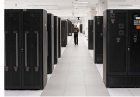
IBM Data Center, Present
