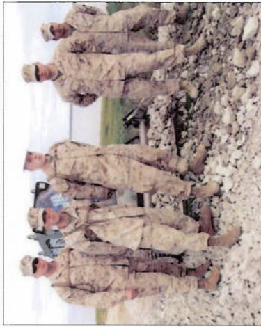
ABOVE: From left: Jason Salemi, Kyle Shokoleva, Cameron Peck of Washington; Jamie Corwin, Brian Guyer of Michigan; and Zach Lande of Idaho work on laying the road's rocky base. TOP: An aerial view of the village site of Mertarvik.
