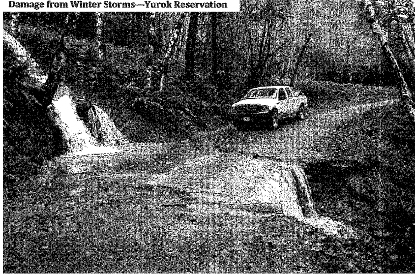
Damage from Winter Storms—Yurok Reservation
