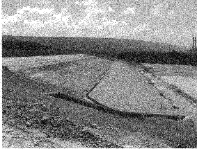
Photo A-3: Completion of Rock Toe Buttress and Preparation of Vegetative Cover Along the West Slope of Gypsum Stack
