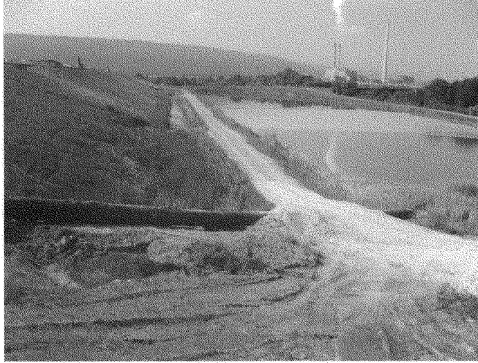
Photo A-1: As Found Site Conditions of the West Slope of Gypsum Stack; Process Water Redirected Through Temporary Spillway Discharge Pipe (foreground)
