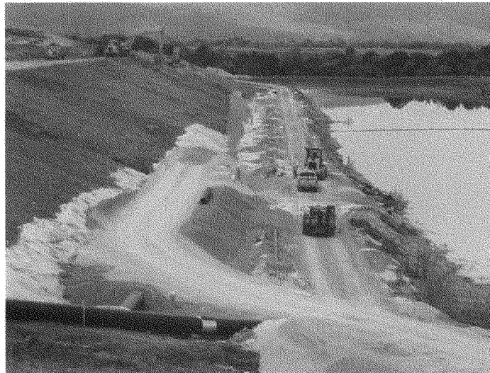
Photo A-2: Construction of Rock Toe Buttress and Spillway Renovations Along West Slope of Gypsum Stack
