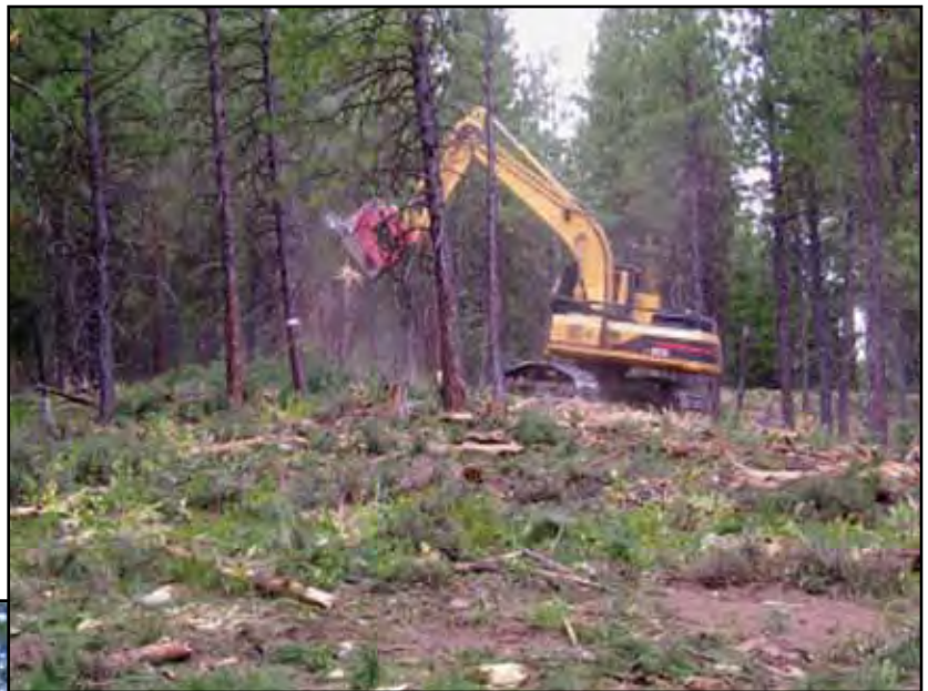
Figure 21. The first entry of a free selection system being accomplished using a masticator. Depending on stand conditions, the majority of the ladder fuels and small trees (less than 20 cm, 8 in) were chunked, leaving a clumpy high forest canopy. The objective of the system is to create and maintain a wildfire resilient ponderosa pine forest located in southern Idaho, similar to those that occurred historically.
