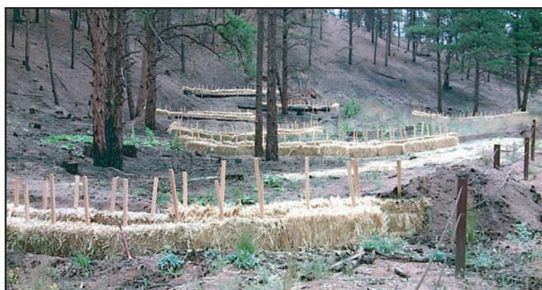
Figure 10. A set of straw bale erosion barriers installed in a burned swale on the 2002 Hayman Fire in Colorado.
