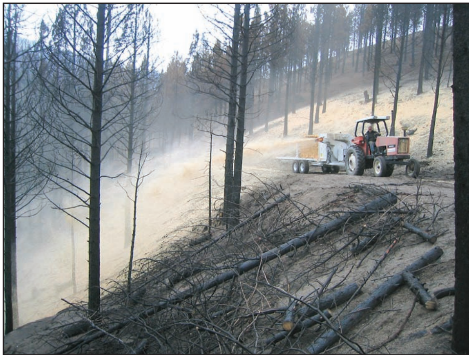
Figure 19. Post-fire straw mulch treatment being applied downslope from a road using a trailer-mounted blower pulled by a tractor on the 2007 Cascade Complex Fires in Idaho.
