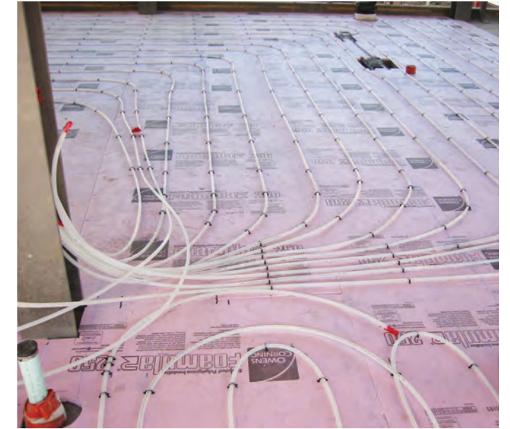
Radiant tubing ready to have 3" thick topping slab poured over it to create a radiant slab floor
