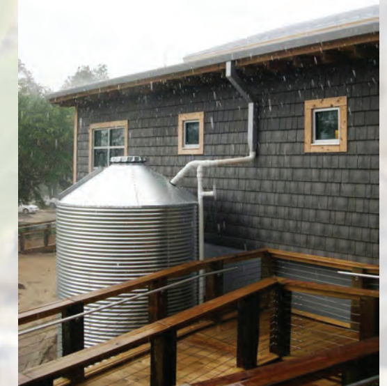
stormwater collection cistern
