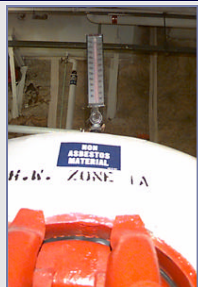
Fig. 2: Thermometer on a storage tank
