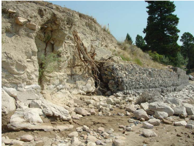
Figure 8. An example of a gabion wall on Canyon Ferry Reservoir with flanking erosion due to deflected wave energy.
