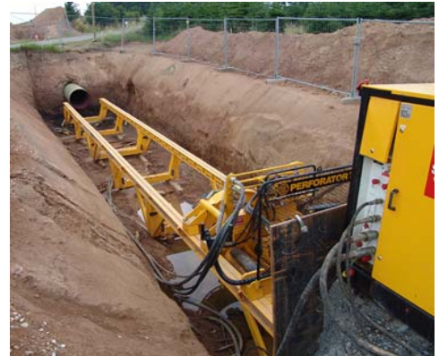
Trenchless construction techniques could be used to avoid disturbing major roadways, streams, and other resources.
