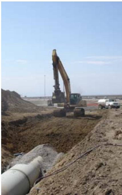
The AVC would be a buried pipeline, typically using open cut installation methods.
