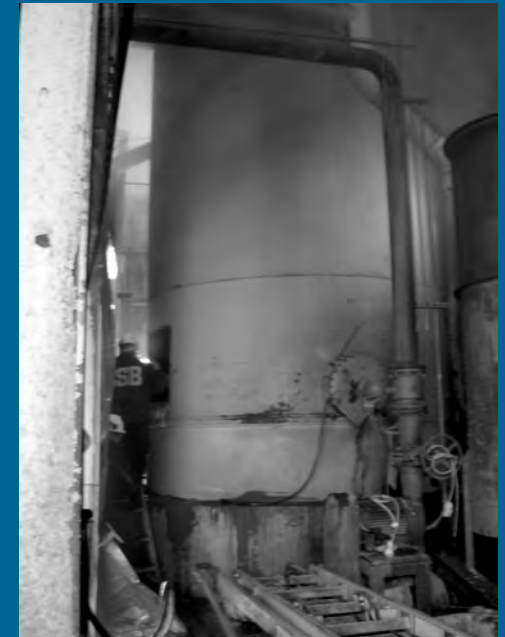
An explosion at the ConAgra Foods potato processing facility in Boardman claimed the life of a welder repairing a leak in a steel tank.
