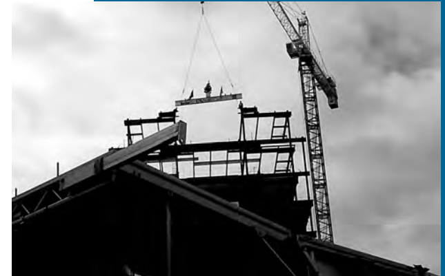
Turner Construction set the final beam before more than 600 guests during the “Topping out Ceremony” at the University of Kentucky Hospital’s Albert B. Chandler Tower construction project.
