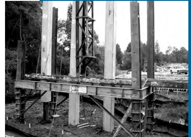
Bridge construction pile driving fatality.
