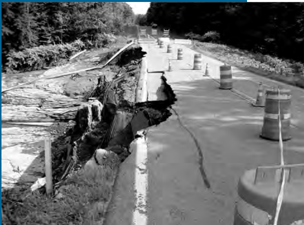
Bridge damage due to water surge from the 2009 Chautauqua County floods.
