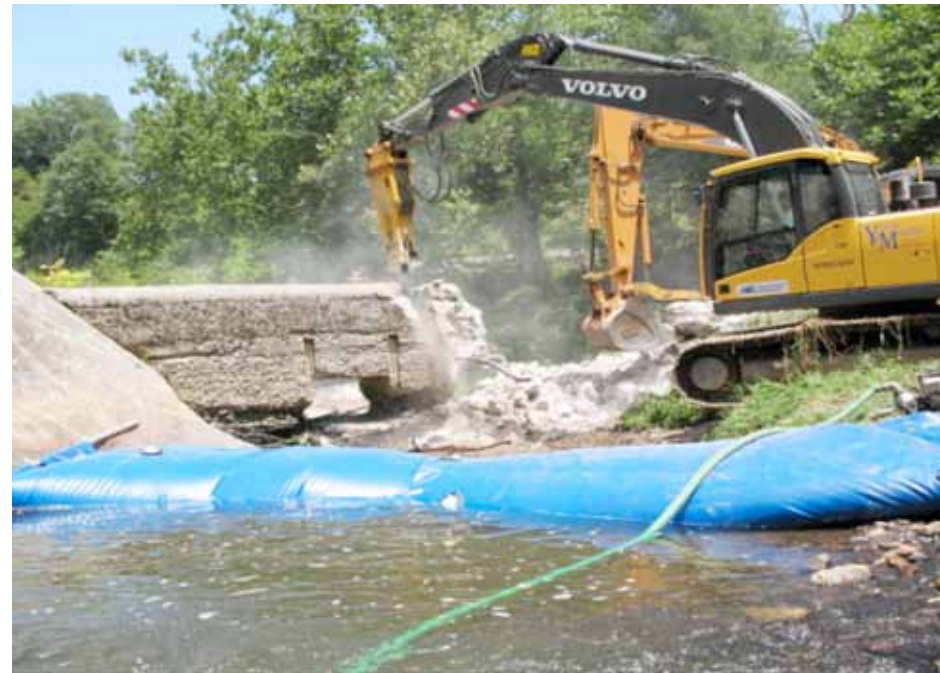
Demolition of the Toe River (Spruce Pine) Dam in the Upper Nolichucky Focus Area. Local contractors use two excavators to remove the dam’s right section. One is equipped with a hydraulic hammer to break up the dam, while another moves rubble out of the way to be disposed of at a later date. This project restored passage for fish and other aquatic species to over 40 miles of the river mainstem, and provided a safer passage for recreational users, USFWS.
