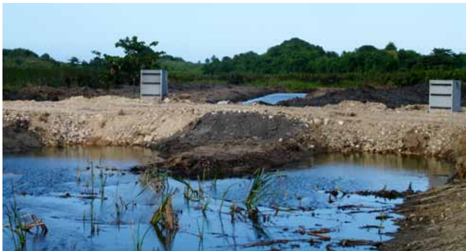
Restoration in freshwater marsh with water-control structures in northern Puerto Rico, USFWS.
