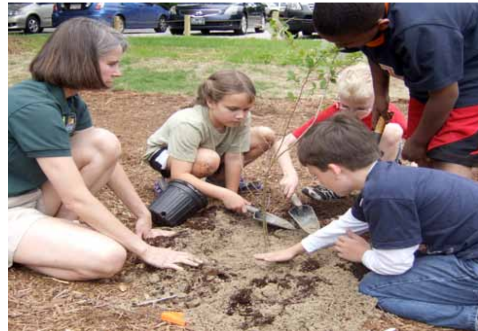
PFW Coordinator John Ann Shearer works with students from AB Combs Leadership Magnet Elementary School in Wake County, North Carolina to plant native plants in a newly constructed rain garden. The rain garden was built to improve water quality in the impaired Simmons Branch watershed by filtering runoff. It will also provide an outdoor learning lab for students and teachers, USFWS.
