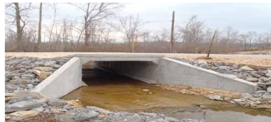
The PFW Program supplies funding to replace existing barrel culverts with concrete box culverts in situations where they form a barrier to slackwater darters returning to their historic spawning areas, USFWS.
