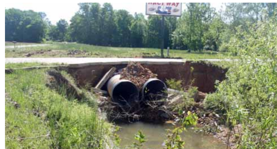
Culverts like the one above prevent slackwater darters from migrating up stream to small headwater reaches where they spawn during late winter, USFWS.
