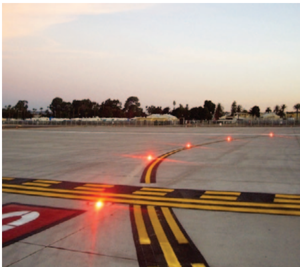
Figure 15 Runway Status Lights
