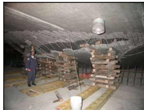
Figure 11. NJ-TF1 cribbing the collapsed section of Tropicana parking garage.
