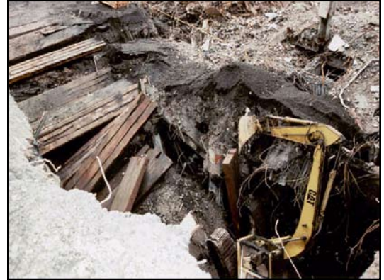
Figure 18. Grappler that fell through surface of pile at WTC. Courtesy of OSHA.
