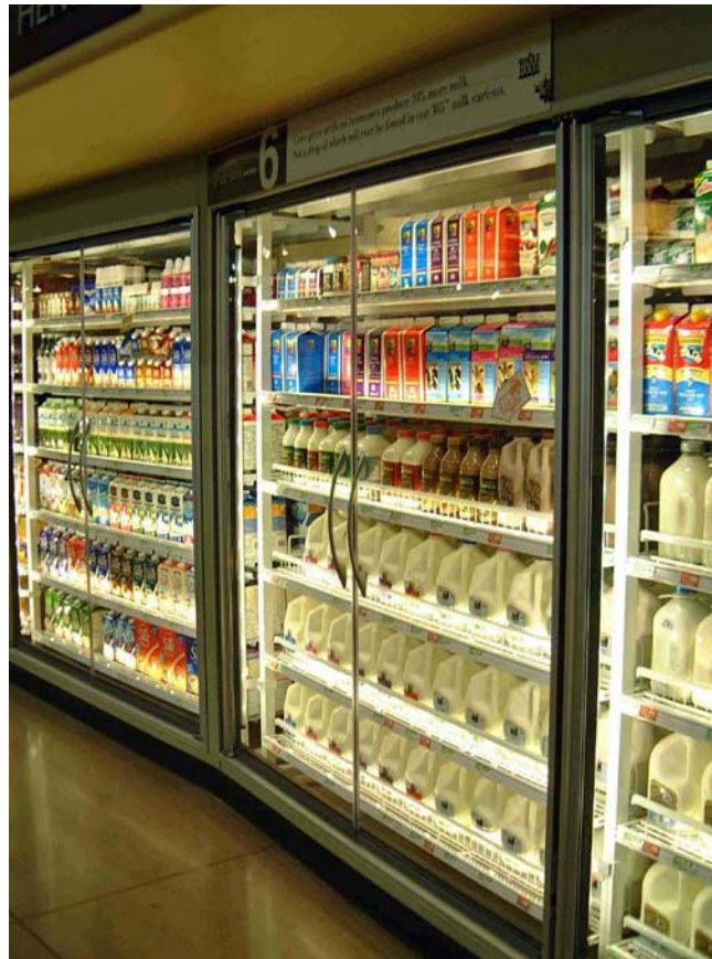
Figure F-3 Doors installed on medium-temperature refrigerated cases at a Whole Foods Market
