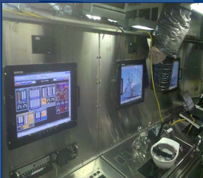
The new engine room of a refurbished 270-foot Medium Endurance Cutter. U.S. Coast Guard photo.
