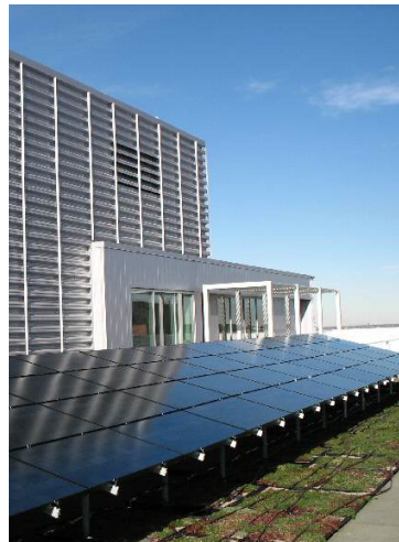
Solar panels on a green roof
