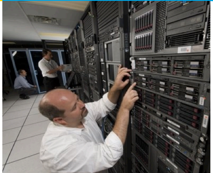
Figure 1. NREL's legacy data center
