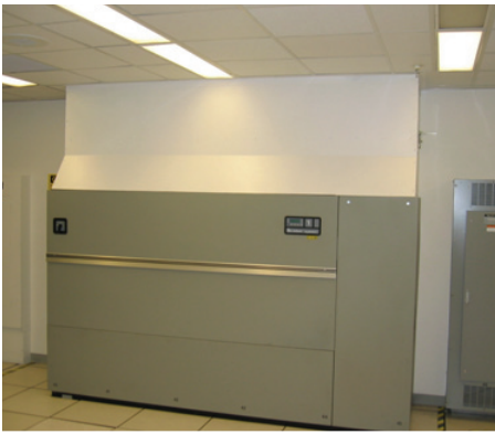
Figure 4: Return duct from plenum to CRAC unit
