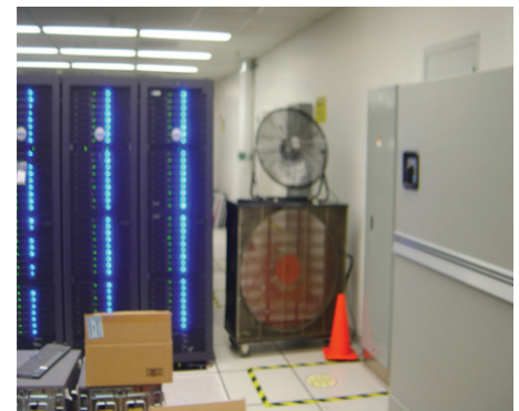
Figure 3: Before retrofit auxiliary fans cool hot spots
