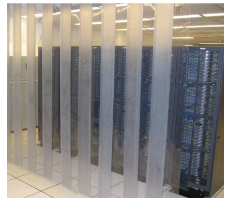
Figure 7: Isolation air curtains with fusible links
