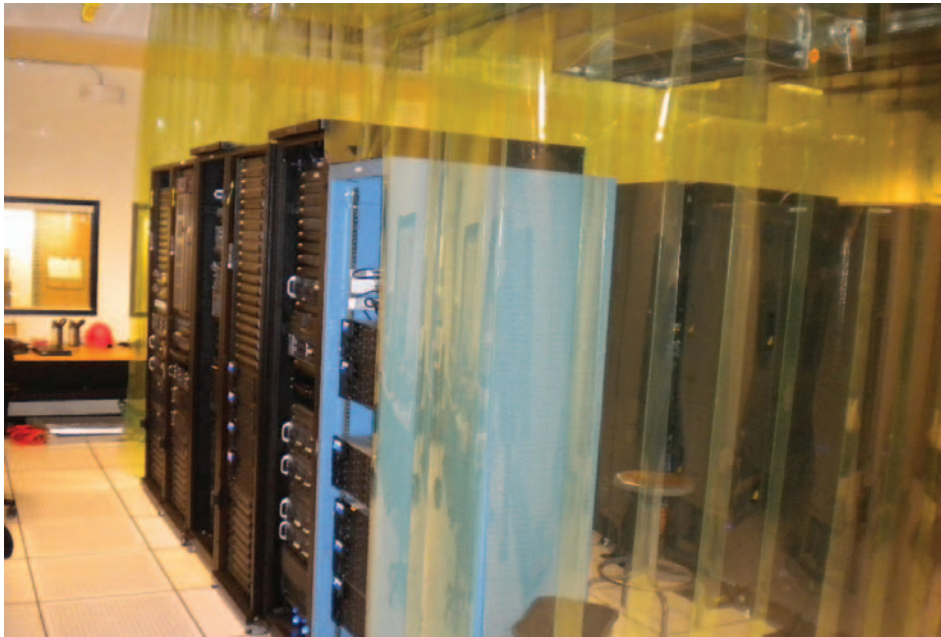
NSIDC hot aisle curtains. Photo used with permission from the National Snow and Ice Data Center.
