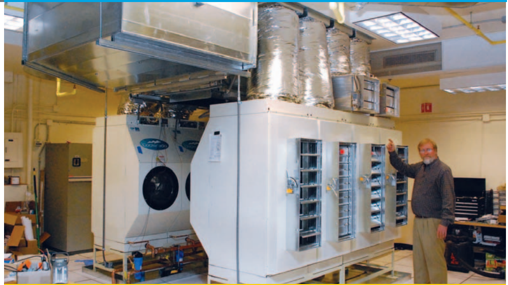
The above photo shows the multi-stage indirect evaporative cooling units installed at the National Snow and Ice Data center in May 2011. Photo used with permission from the National Snow and Ice Data Center.
