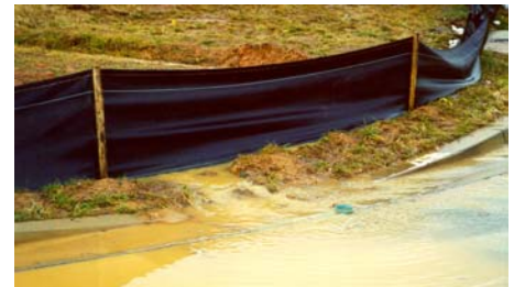
An example of improper trenching
