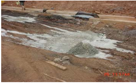
Improper concrete washout near storm drain with no protective barriers
