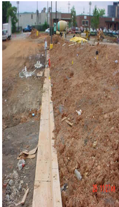
Improper soil stabilization
