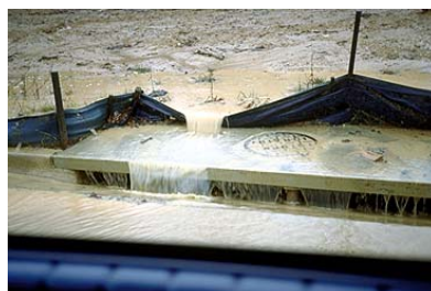
Silt fence failure overwhelms storm drain
