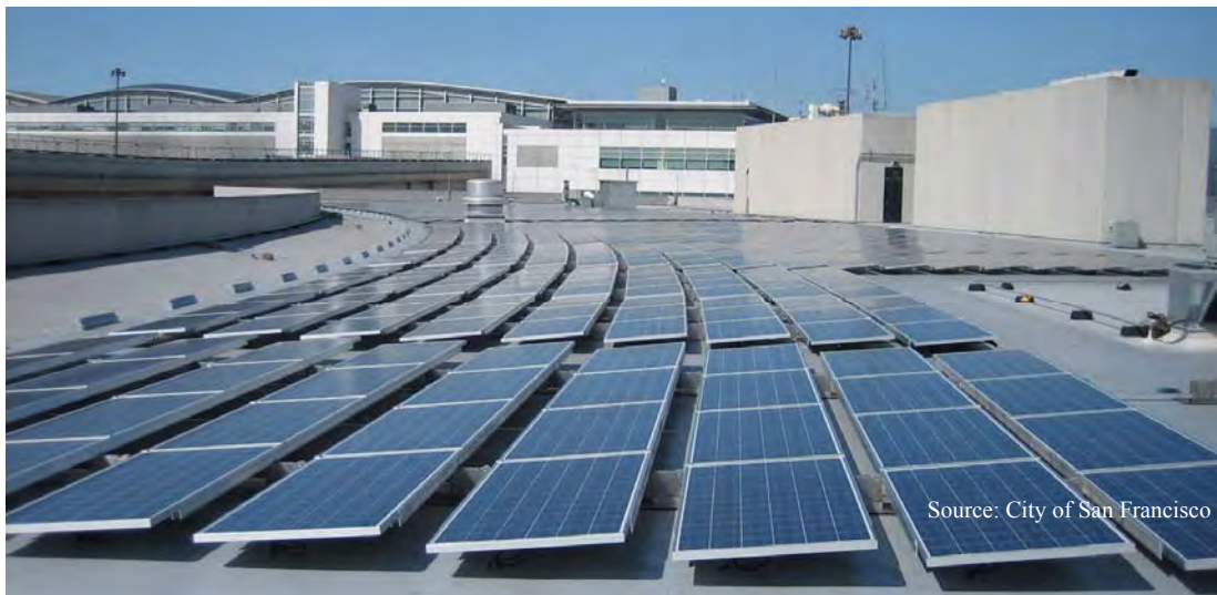
Figure 25: Rooftop Solar Project on San Francisco's Terminal 3
