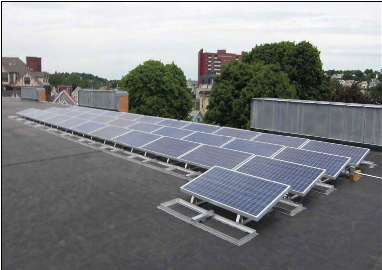
Figure 6: Example of a Roof-Mounted Solar PV System
