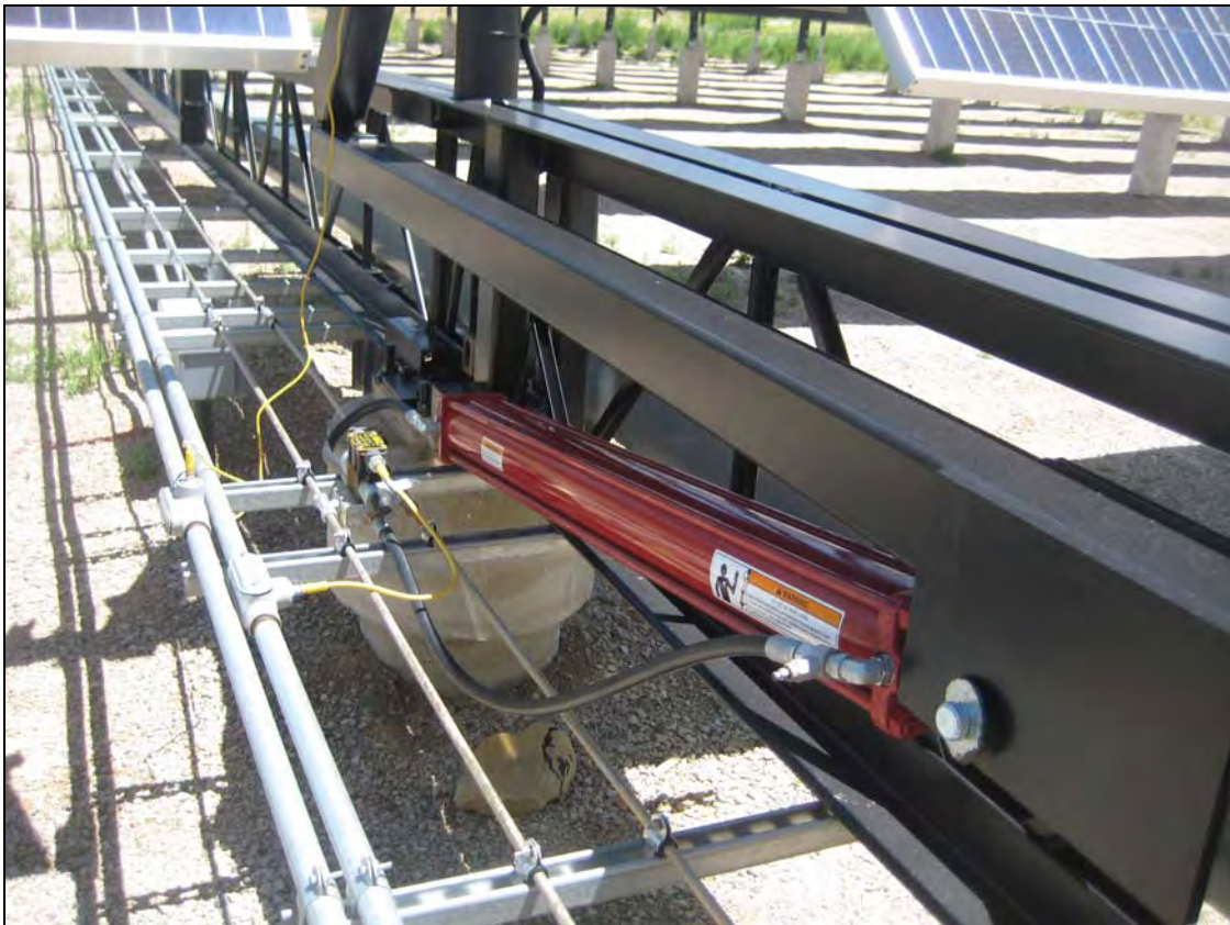
Figure 8: Example of a Tracking Solar PV Installation
