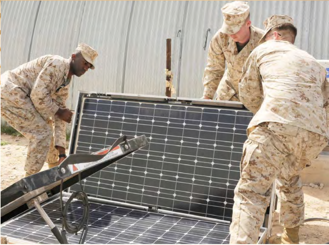
Marines set up the Ground Expeditionary Energy Network System, a joint venture by the Navy and Marine Corps to find alternate power systems to decrease the dependability, on Camp Tombstone in Helmand province, Afghanistan. DLA Energy assists bases, installations, laboratories and other federal and military locations seeking on-site renewable energy generation. Photo by Marine Sgt. Laura Bonano
