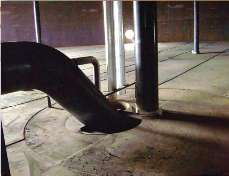
A tank's sump and 24-inch issue line are installed at a defense fuel support point at Point Loma, Calif., as a part of its military construction efforts. Fuel above the flange is issuable fuel. Once it falls below the flange, the pipe loses suction and the piping in the sump allows the fuel to be drained.
