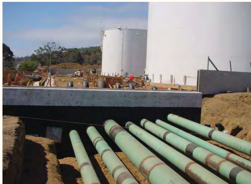
Piping rigging that will go around new tanks at Defense Fuel Support Point Point Loma, Calif., is installed as a military construction effort P-401 rebuilds the facility after it reached the end of its lifecycle.
