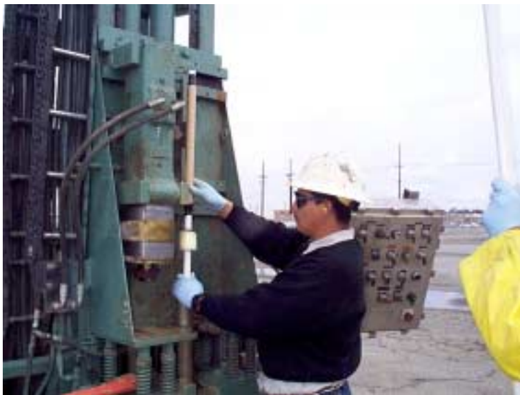
Image 10. Installation of \frac{3}{4} -inch direct-push no filter pack well consisting of an expandable bentonite sleeve above the screen.
