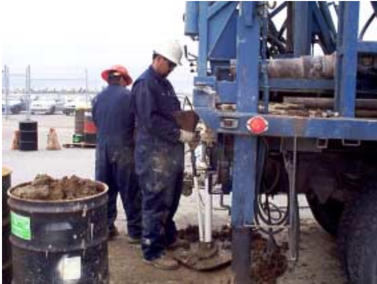
Image 5. Tremmie installation of a filter pack for a 2-inch diameter well installed using a hollow stem auger drilling technique.
