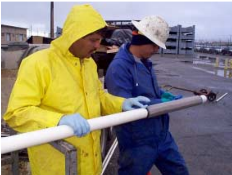
Image 6. Preparation of a 2-inch diameter direct-push monitoring well with a prepacked filter.
