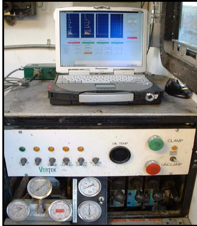
Figure 2-12. Data acquisition system laptop with software on operator control console.
