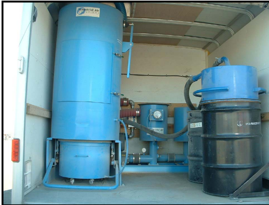
Figure 2-13. Air filtration equipment in support trailer. Cyclone separator (right), bag filter (left), HEPA and carbon filters (background).
