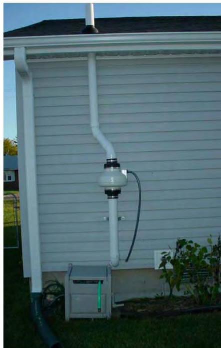
Figure 3b. Actual Vapor Intrusion Mitigation System (ITRC 2007)
