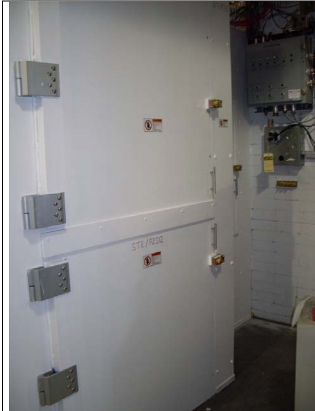
Figure 2: Small Transport Enclosure (STE) downstream access door/panels
