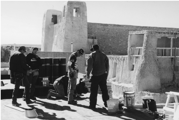
The gaugashti (caretaker of the church) with Acoma crew restoring the meeting house.
