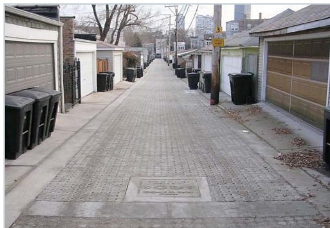
Figure 10: Chicago's Green Alley program retrofits existing alleys to include permeable pavers as seen in this residential alley. Photo courtesy of David Leopold.
